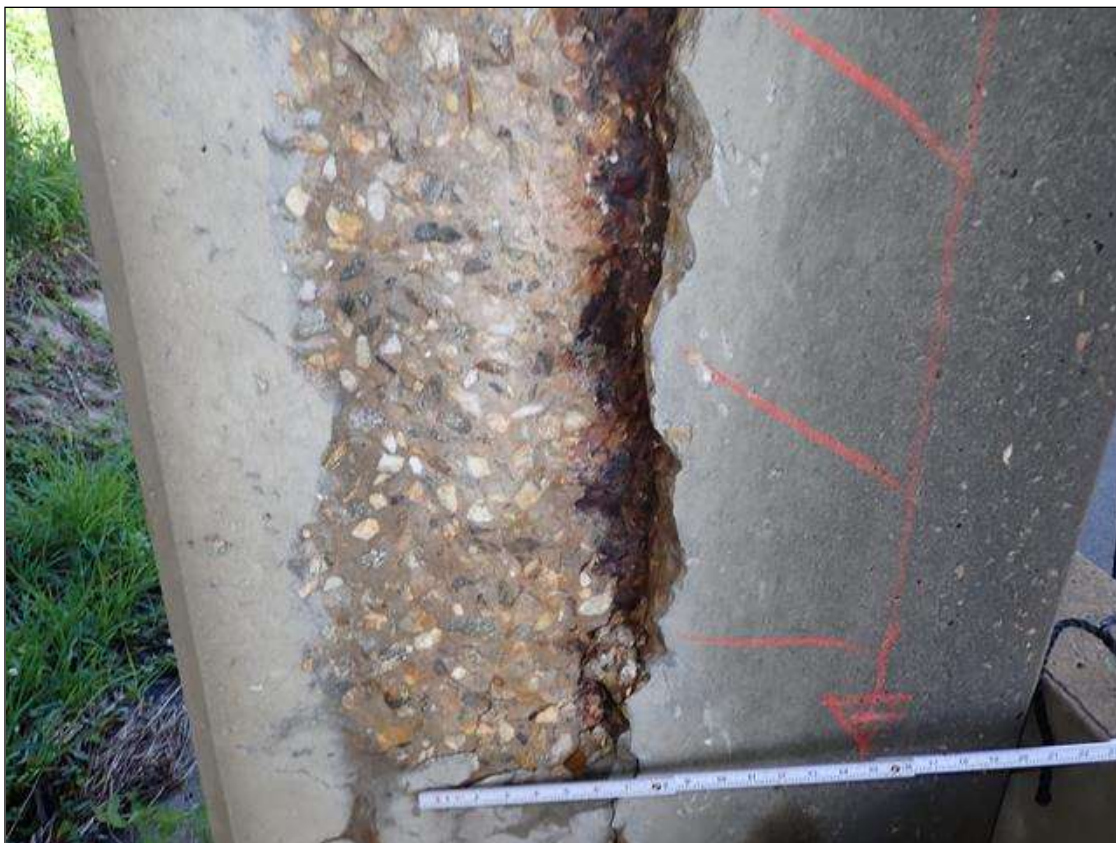
Bent 3 Pile 3: (PAR) west face, spall/delamination (20 inch x full height x 2 inch deep) with exposed rusted rebar (approximately 25 percent loss) and cracks (up to 1/8 inch) some with efflorescence
