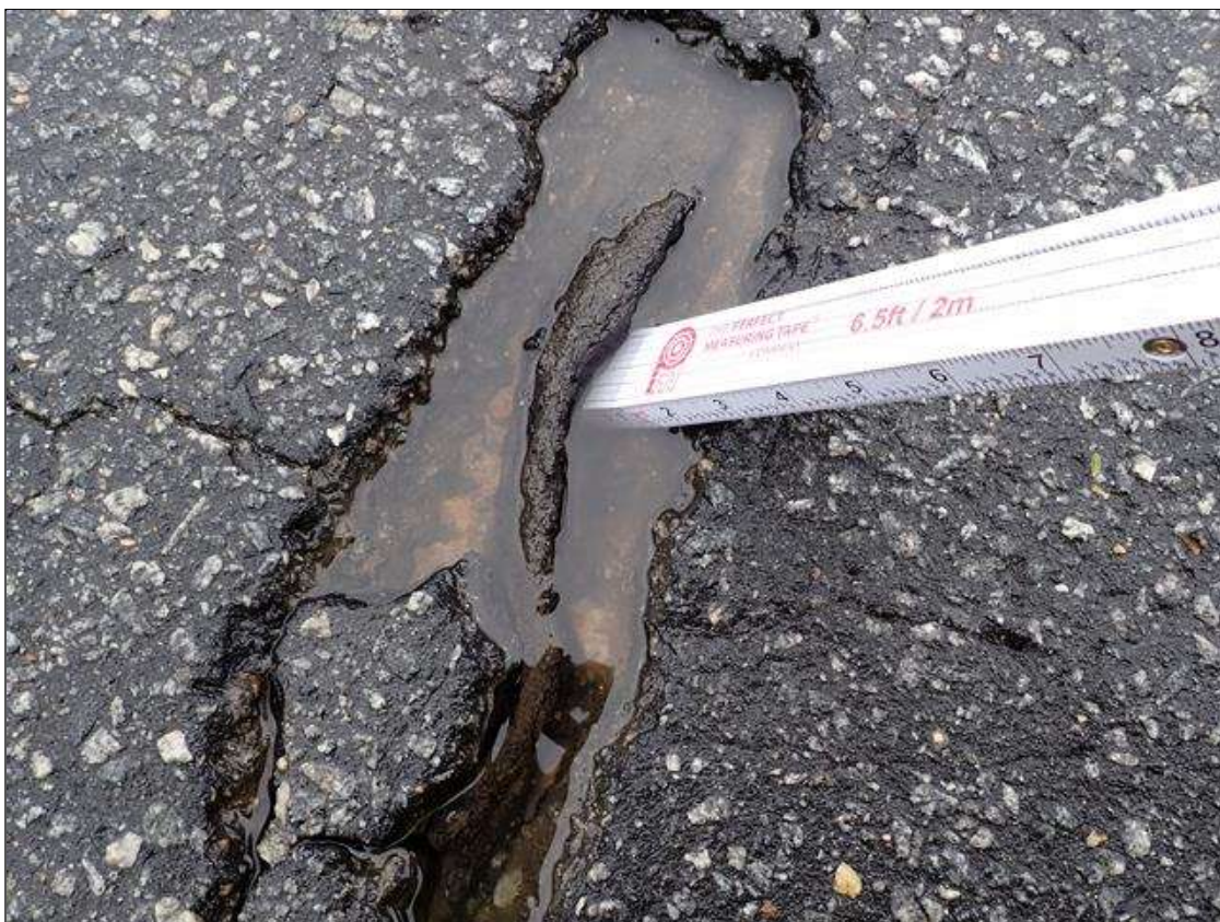
Span 2 Bent 1 Expansion Joint: at missing asphalt locations, seal deteriorated/torn/missing (up to full depth)
