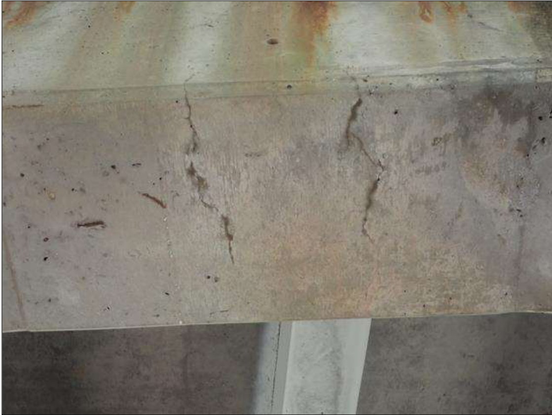
Bent 2 Cap 1: along the length of the cap, vertical cracks (up to 1/32 inch x full height) some extending into bottom face (full width) and map cracks (hairline) at random
