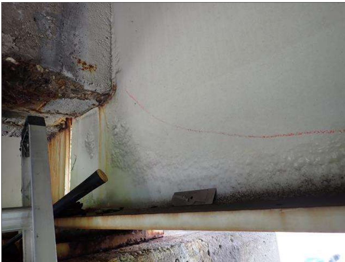
Span 2 Beam 5: at bent 2, painted over pitting: web (up to 1/8 inch deep x 10 foot x 24 inch); bottom flange, painted over section loss (0.70 inch average remaining x 10 inch); bottom flange 10 inch from bearing, painted over pitting (up to 1/16 inch pitting x 10 foot)
