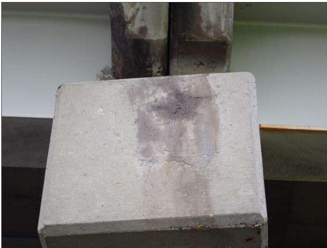
Bent 1 Cap 1: 8 INCH DIAMETER PATCH, IN WEST END OF CAP.
