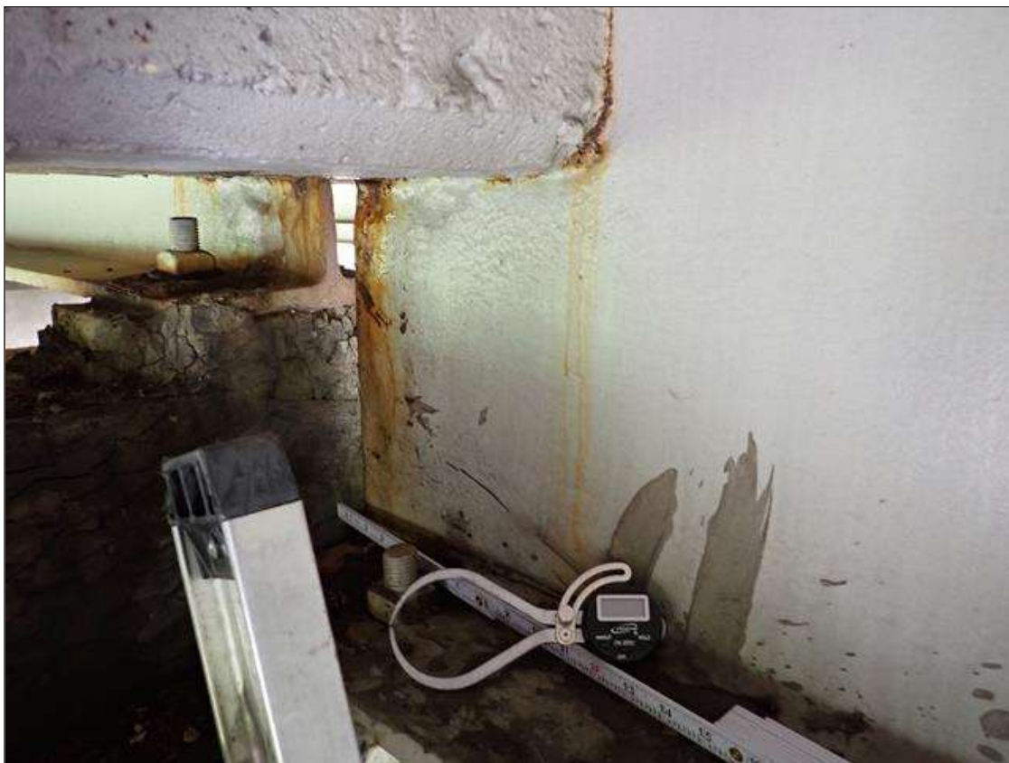
Span 2 Beam 3: (PAR) at bent 1, painted over section loss/pitting: web adjacent to end diaphragm ( 3/8 inch average remaining x 2 inch x 8 inch); bottom flange, pitting (up to 1/16 inch deep x 2 foot); web, pitting (up to 1/16 inch deep x 2 foot x up to full height)
