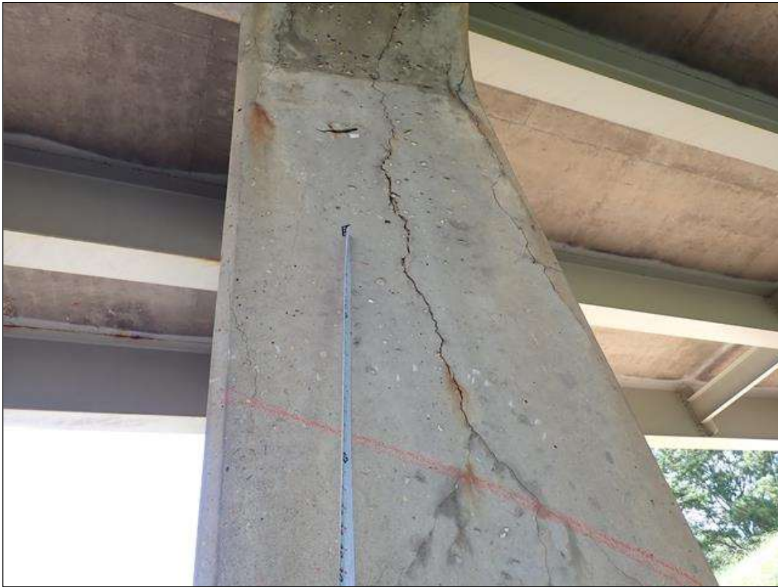
Bent 3 Pile 2: (PAR) east face below cap, delamination (full width x 5 foot) with cracks (up to 1/8 inch) with rust stains
