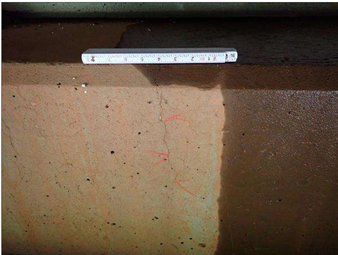
End Bent 2 Cap 1: END BENT 2 CAP HAS SCATTERED CRACKS THROUGHOUT ALL BAYS, UP TO TO FULL HEIGHT X 1/32 INCH
