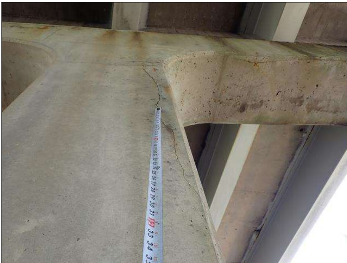
Bent 2 Pile 2: northwest and southwest corners below cap, (3) delamination (4.5 foot x 1 foot) with cracks (up to 1/16 inch)
