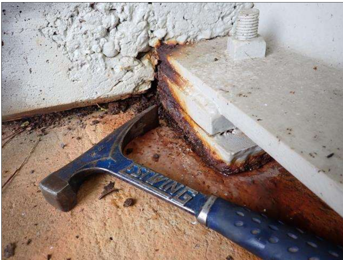
Span 4 Beam 1 - Far Bearing 1: corrosion with section loss (up to 1/8 inch loss)
