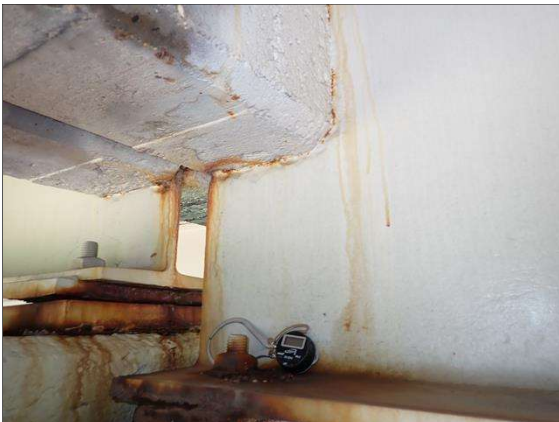
Span 3 Beam 4: at bent 3, painted over section loss/pitting: web adjacent to end diaphragm (1/2 inch average remaining x 10 inch x 2 inch)
