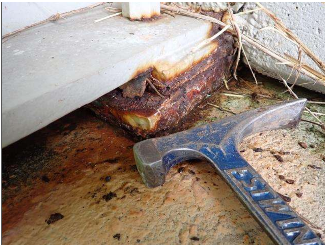
Span 1 Near Bearing 5: corrosion with section loss (up to 1/8 inch loss)
