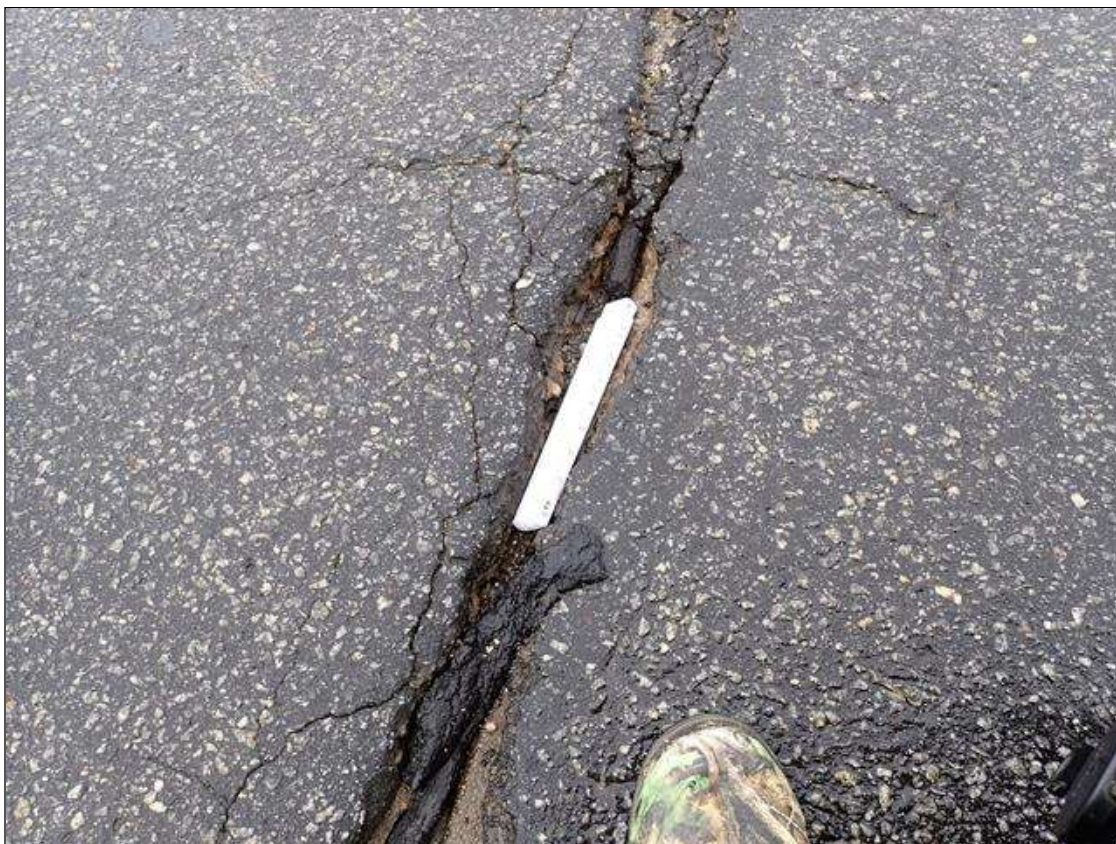
Span 3 Bent 2 Expansion Joint : at missing asphalt locations, seal deteriorated/torn/missing (up to full depth)
