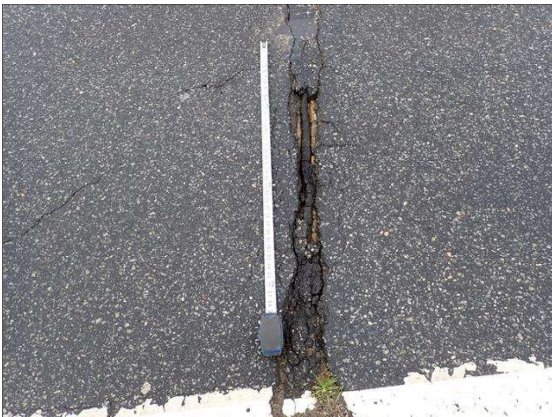
Span 3 Wearing Surface: (PAR) over bent 3, broken asphalt (full roadway width x 8 inch) with potholes (up to 5 foot x 5 inch x full depth)
