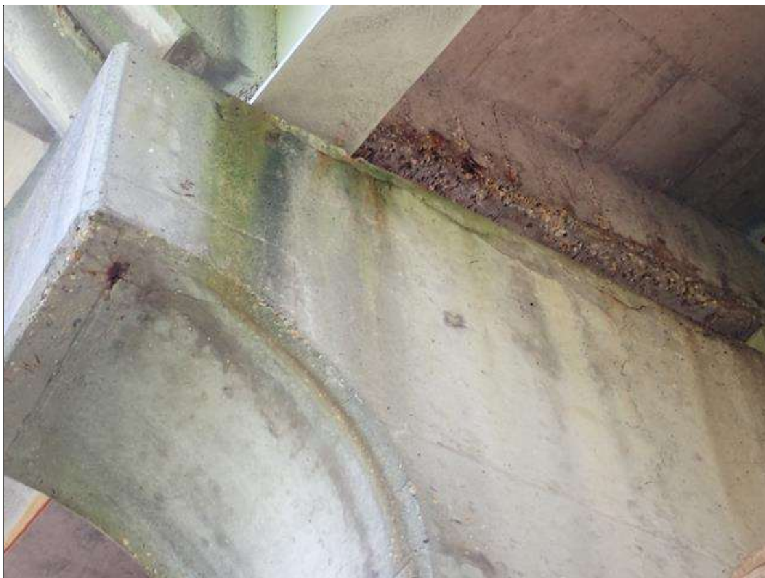
Bent 3 Cap 1: (PAR) both faces and underside, multiple delaminations (15 foot x 18 inch) with cracks (up to 1/8 inch) some with rust stains
