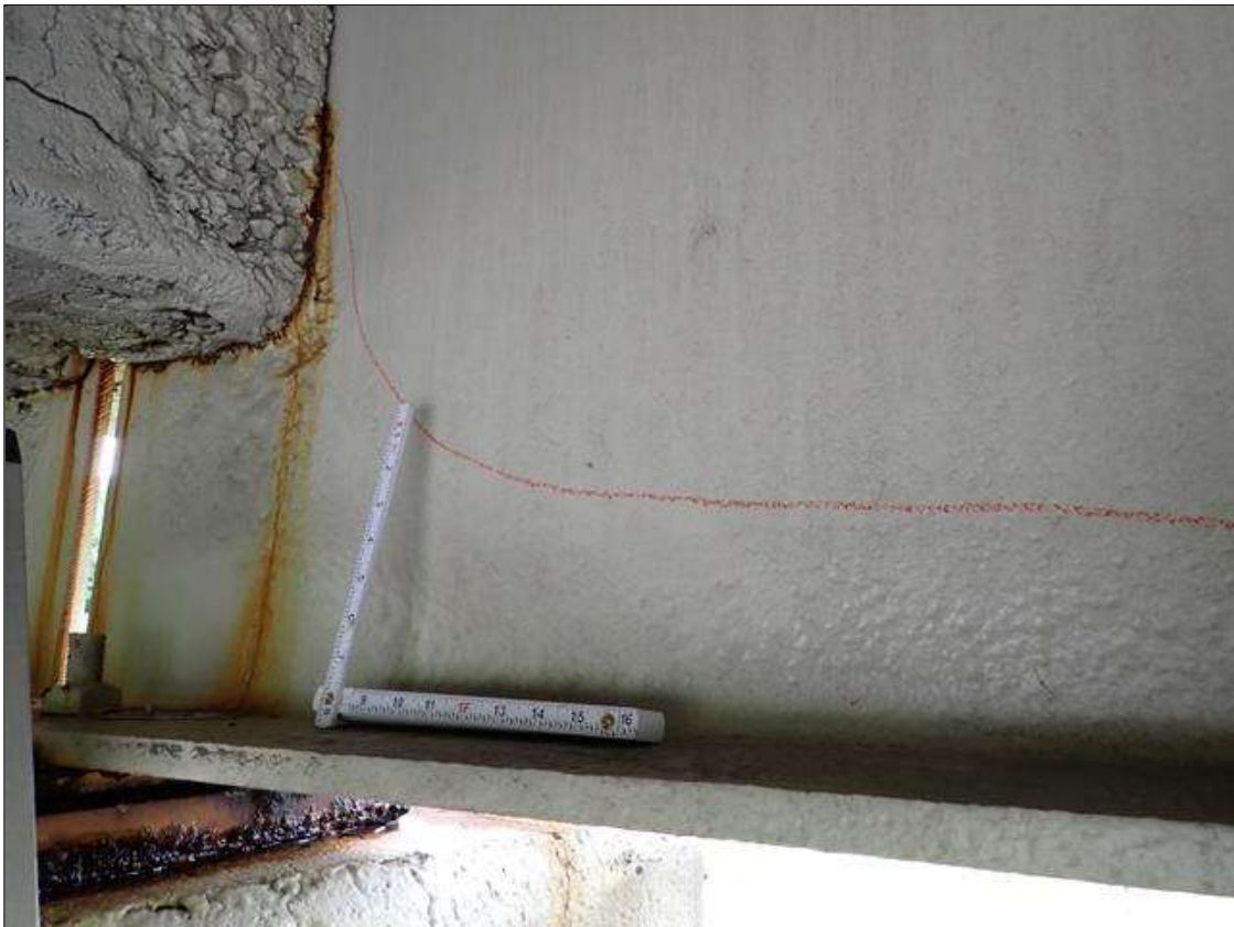
Span 2 Beam 1: at bent 1, painted over pitting: web (up to 1/8 inch deep x 3 foot x up to 17 inch); bottom flange (up to 1/16 inch deep x 3 foot) with corrosion reactivating
