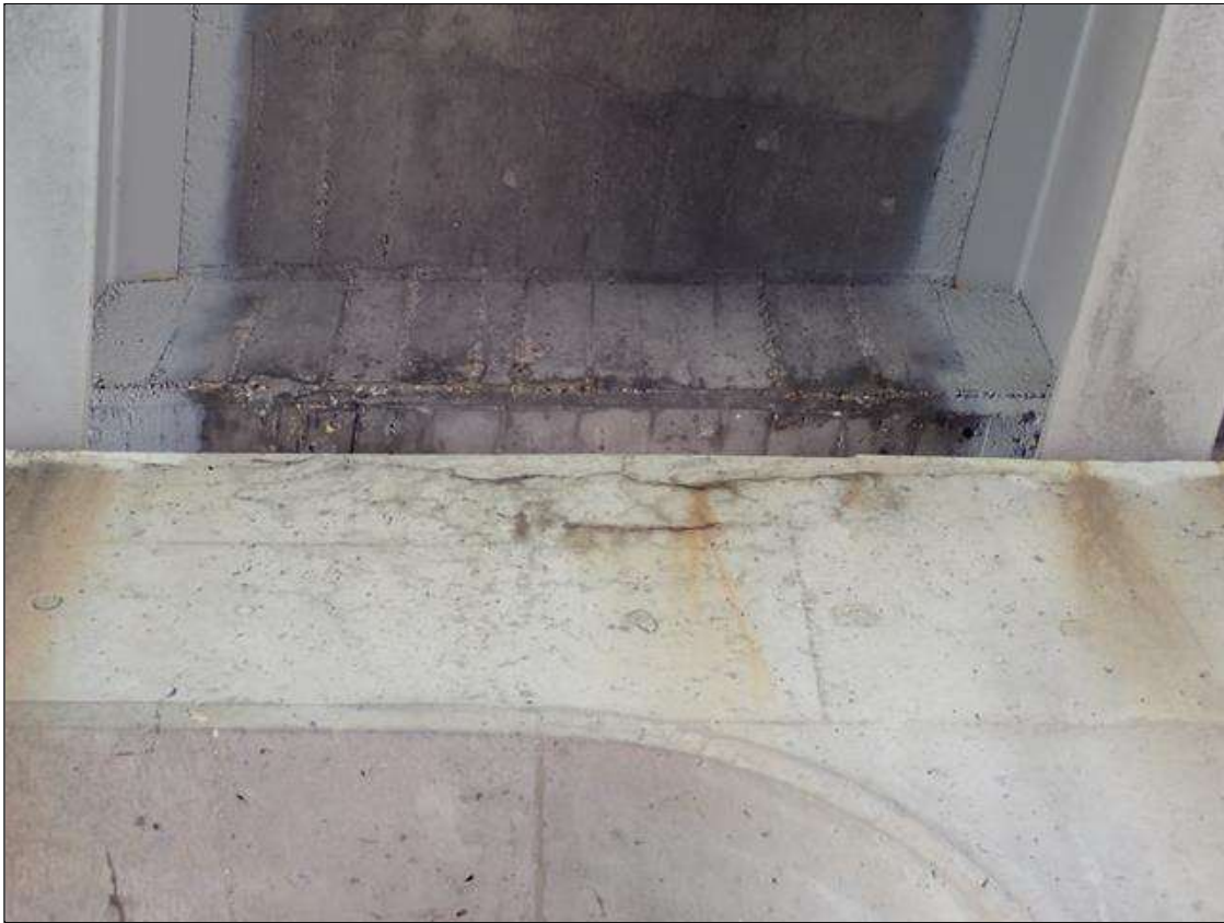
Bent 2 Cap 1: (PAR) UP TO 7 FOOT X 12 INCH DELAMINATIONS WITH HORIZONTAL CRACKS UP TO 1/16 INCH WITH RUST STAINING, SOUTH AND NORTH FACES, UNDER BAY 3.
