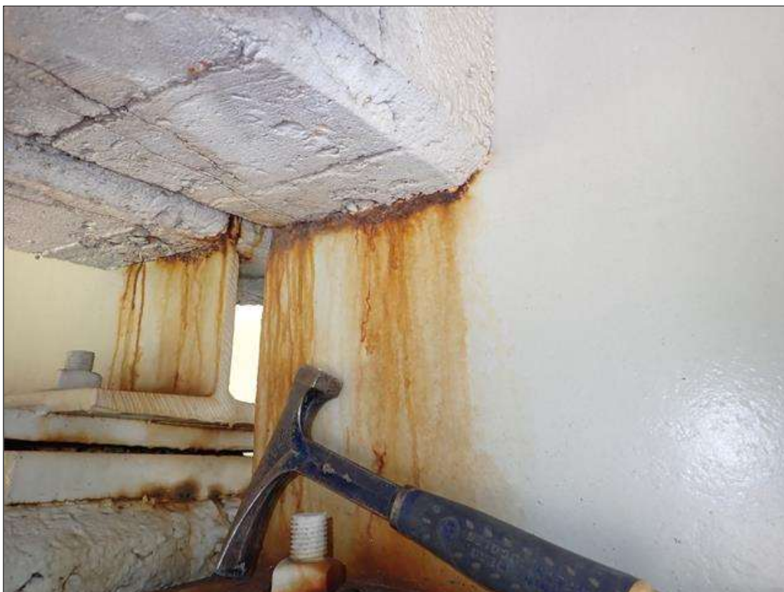
Span 3 Beam 2: at bent 3, web adjacent to end diaphragm, rust scale (10 inch)
