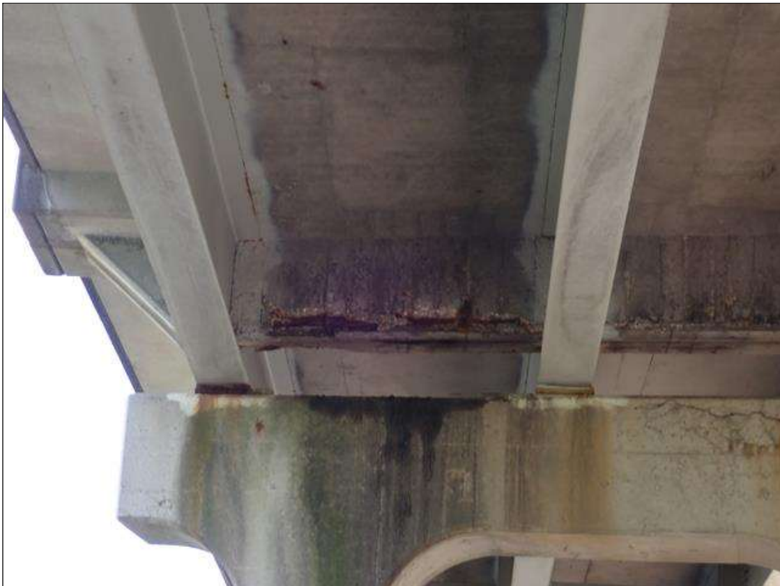
Span 3 Deck: (PAR) bay 4 end diaphragm over bent 2, spalls/delamination (full width x 1 foot x 1 inch deep) with exposed rusted rebar (approximately 25 percent loss)
