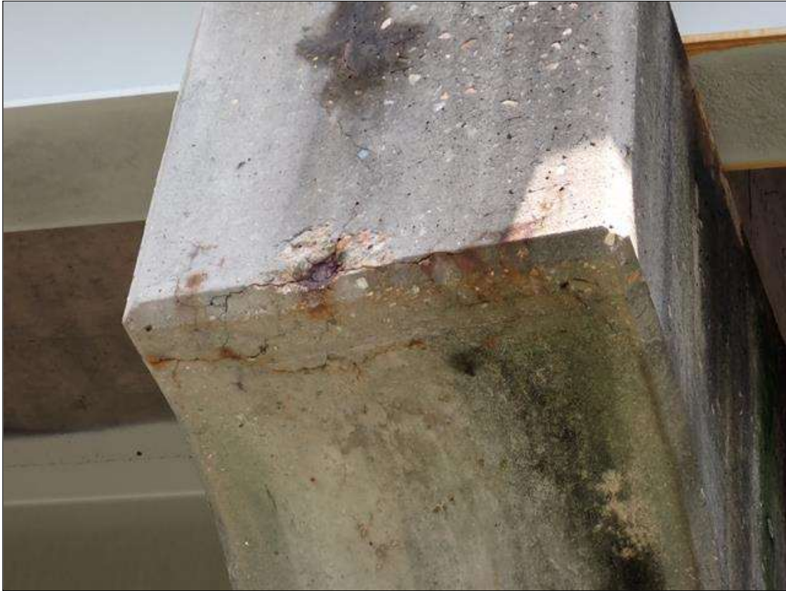
Bent 2 Cap 1: (PAR) BENT 2 CAP WEST FACE BOTTOM CORNER HAS A SPALL AND DELAMINATED AREA (2.5 FOOT X 1 FOOT X 1 INCH DEEP) WITH REBAR EXPOSED (APPROXIMATELY 25 PERCENT LOSS) AND MAP CRACKS (UP TO 1/16 INCH) WITH RUST STAINS
