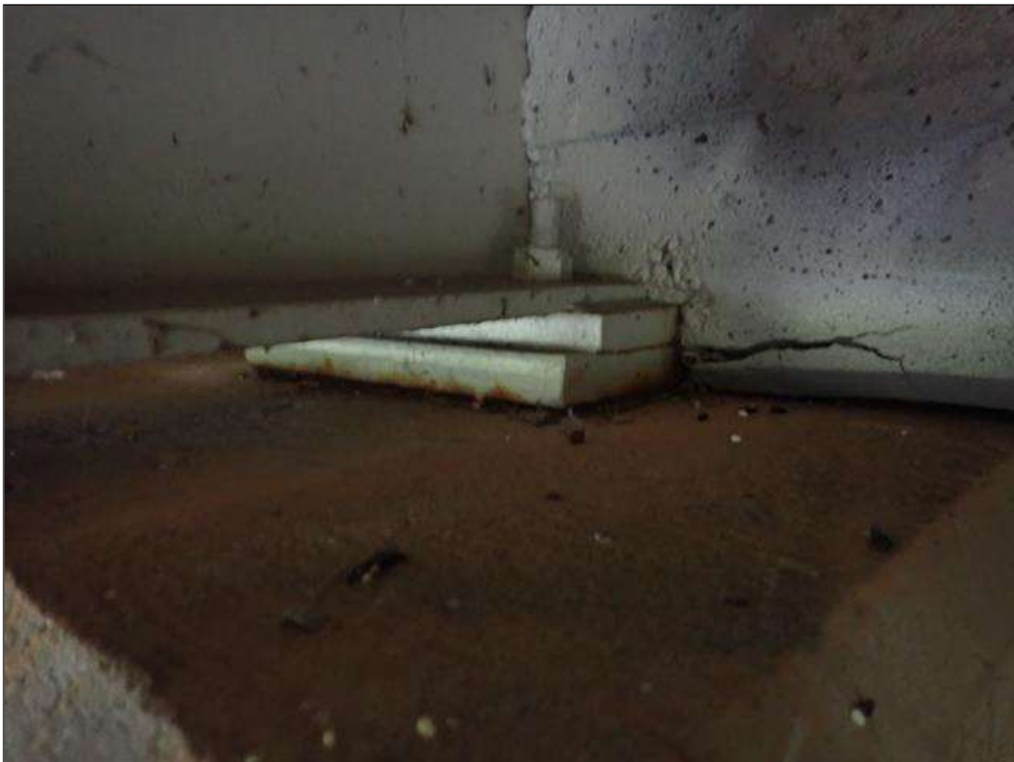
end bearing assembly
