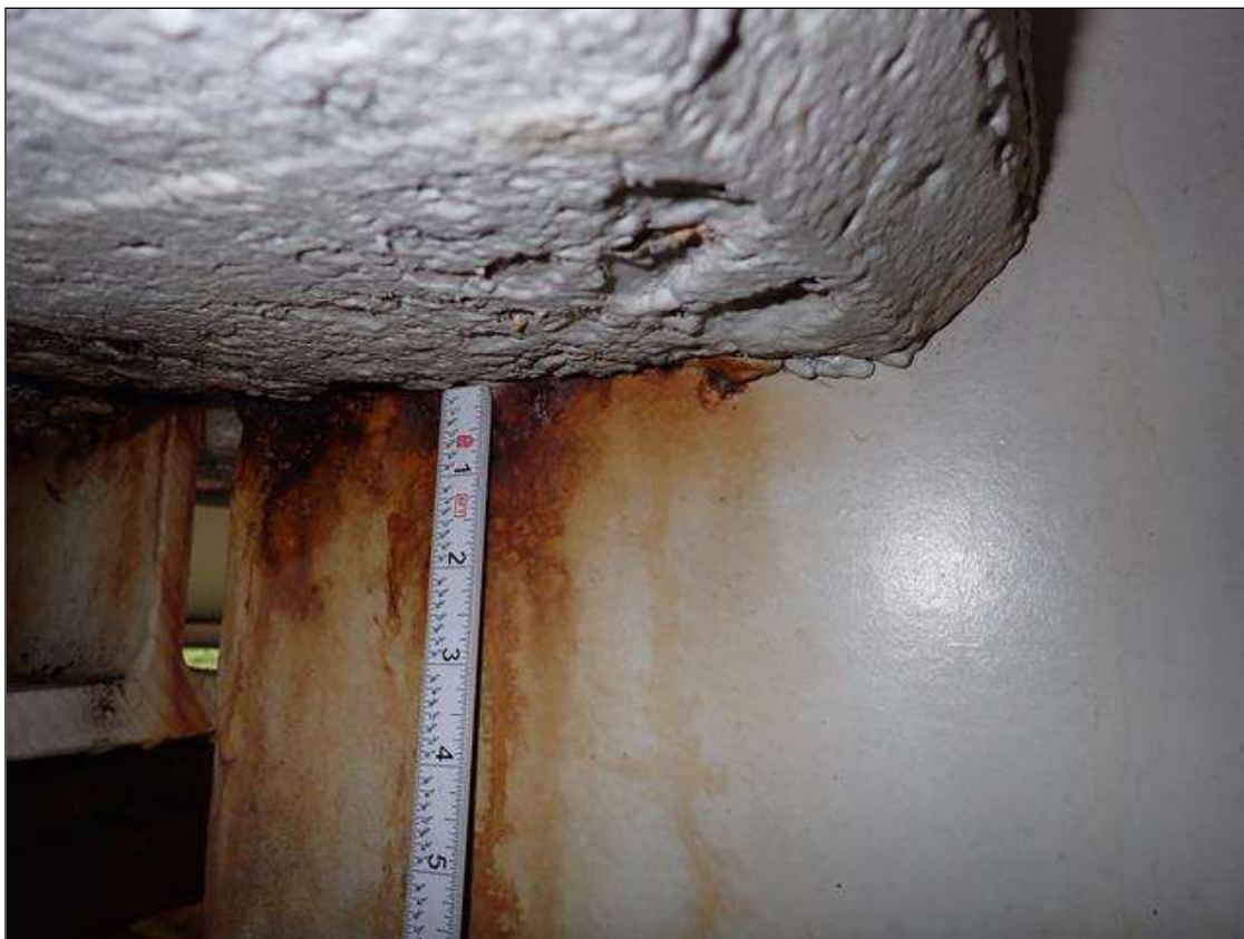
Span 2 Beam 4: at bent 1, painted over section loss/pitting: web adjacent end diaphragm (1/2 inch average remaining x 6 inch x 2 inch)
