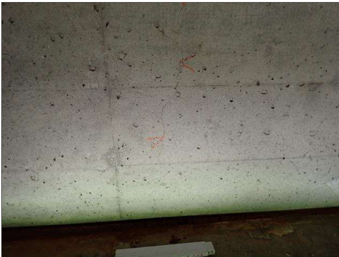
End Bent 1 Abutment: along the length of the abutment, vertical cracks (up to 1/64 inch x full height) at random
