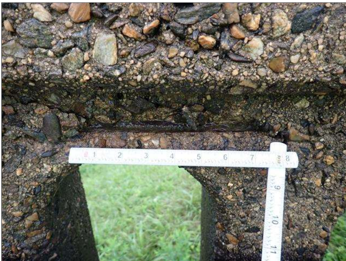
Span 1 Right Bridge Rail: UP TO 6 INCH X 3 INCH X 1/4 INCH DEEP SPALL WITH EXPOSED REBAR AT RANDOM THROUGHOUT
