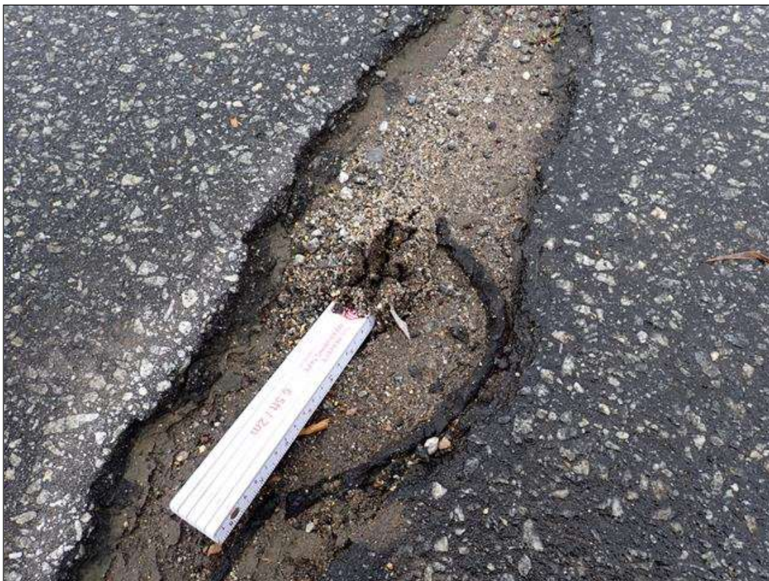
Span 3 Bent 2 Expansion Joint : at missing asphalt locations, debris accumulation (up to full length)
