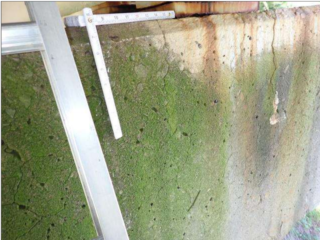
Bent 3 Cap 1: along the length of the cap, vertical cracks (up to 1/32 inch x full height) and map cracks (hairline) at random
