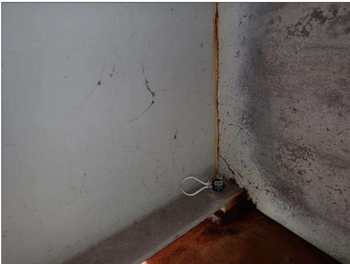
Span 4 Beam 1: (not found 2023) web at far end East face, arrested metal loss, up to 10 inch high x 12 inch long, average remaining 1/2 inch
