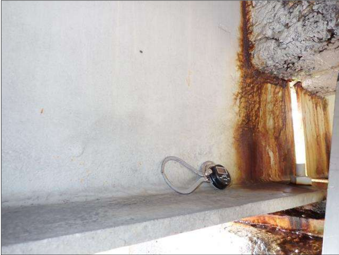
Span 2 Beam 5: (PAR) at bent 1, painted over section loss/pitting: bottom flange (0.72 inch average remaining x 2.5 foot); web (7/16 inch average remaining x 2.5 foot x 18 inch) with corrosion reactivating
