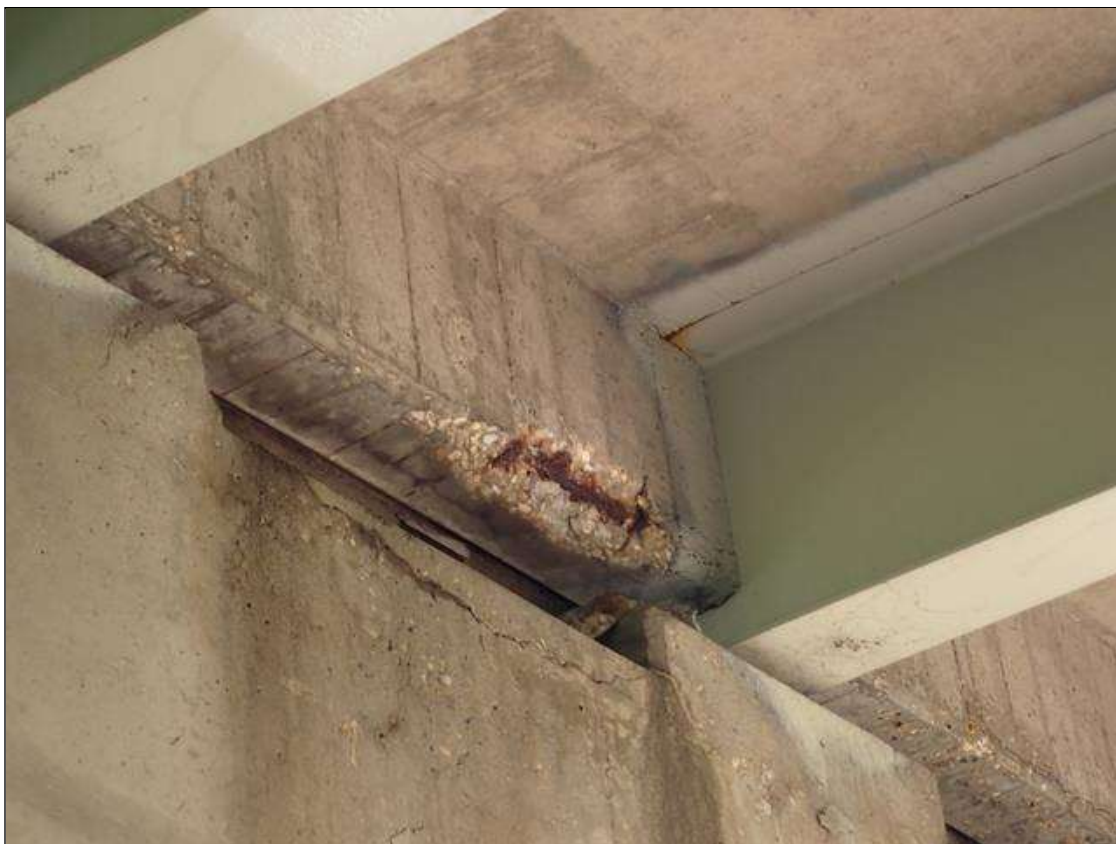
Span 4 Deck: (PAR) bay 2 end diaphragm over bent 2, spalls/delaminations (3 foot x 12 inch x 1 inch deep) with exposed rusted rebar (approximately 25 percent loss)
