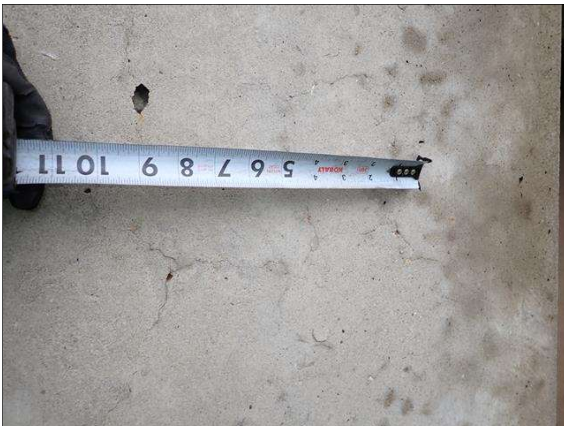
Bent 1 Pile 1: below cap, all corners, delaminations (9 inch x 4 foot) with cracks (up to 1/8 inch); along column, map cracks (hairline) and vertical cracks (up to 1/32 x full height) at random
