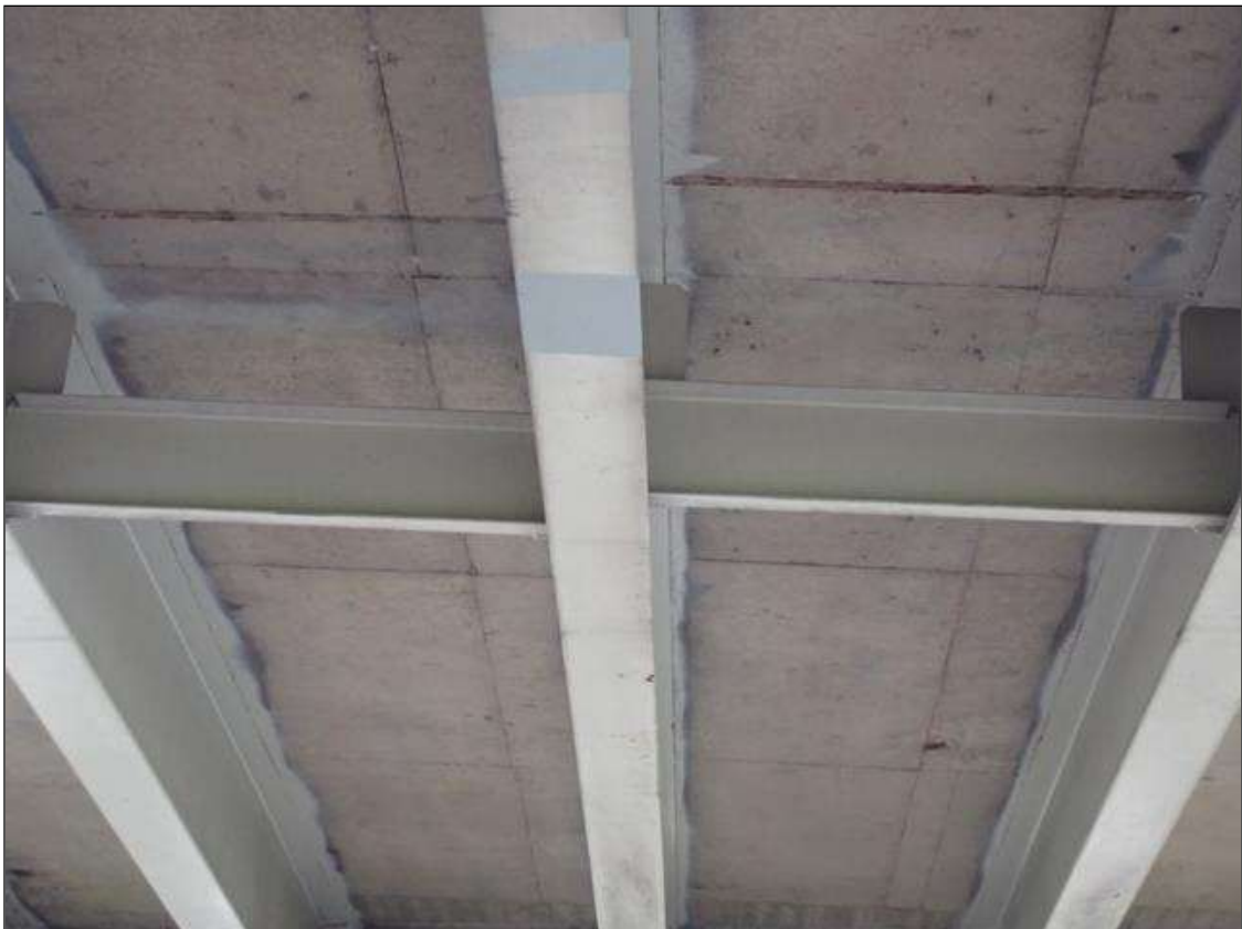
Span 2 Beam 3: SCATTERED SCRAPES TO BOTTOM FLANGE AT RANDOM
