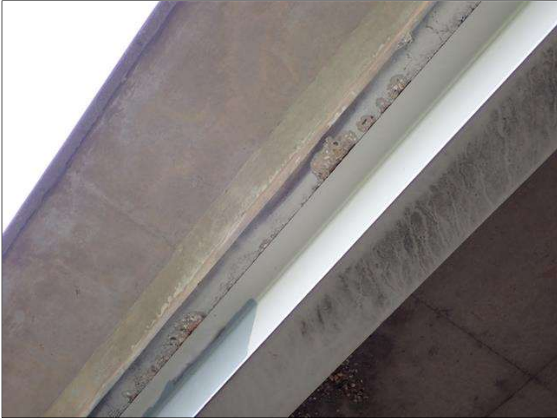
Span 2 Deck: SCATTERED POPOUTS IN BOTTOM DECK AT LEFT SIDE OF TOP FLANGE OF BEAM 1 UP TO 1 INCH DEEP
