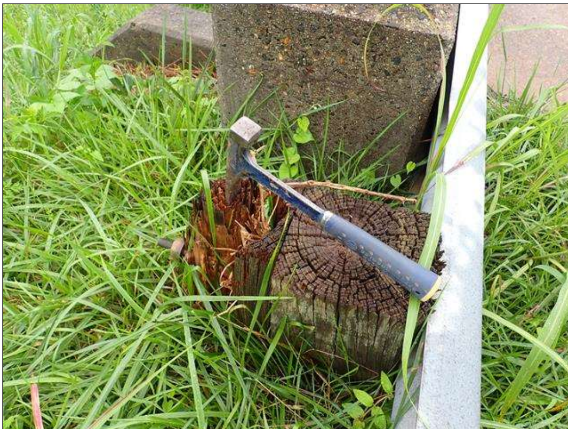
(PAR) southwest guardrail, timber posts 1-5, decay/section loss (up to full width x full height x full depth)
