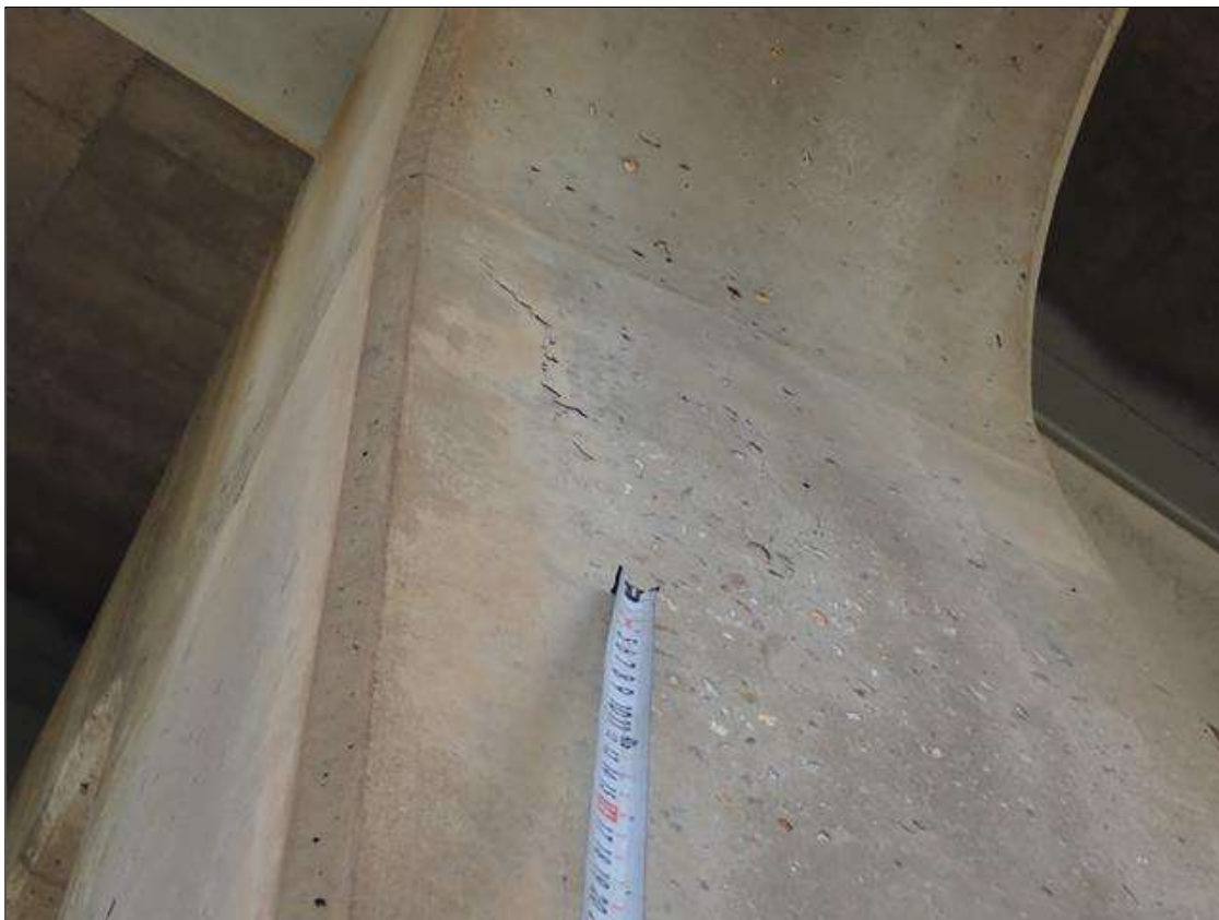
Bent 2 Pile 2: East face below cap, delamination, 32 inch x 11 inch
