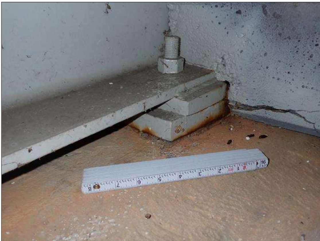
Span 4 Far Bearing 4: surface rust
