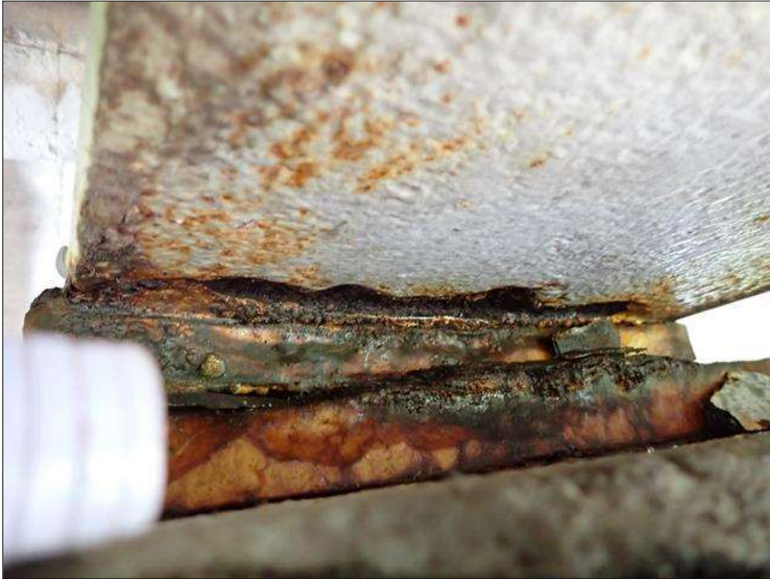
Span 2 Beam 4: at bent 2, painted over section loss/pitting: bottom flange (0.70 inch average remaining x 1.5 inch); web adjacent to end diaphragm (1/2 inch average remaining x 10 inch x 2 inch) with corrosion reactivating
