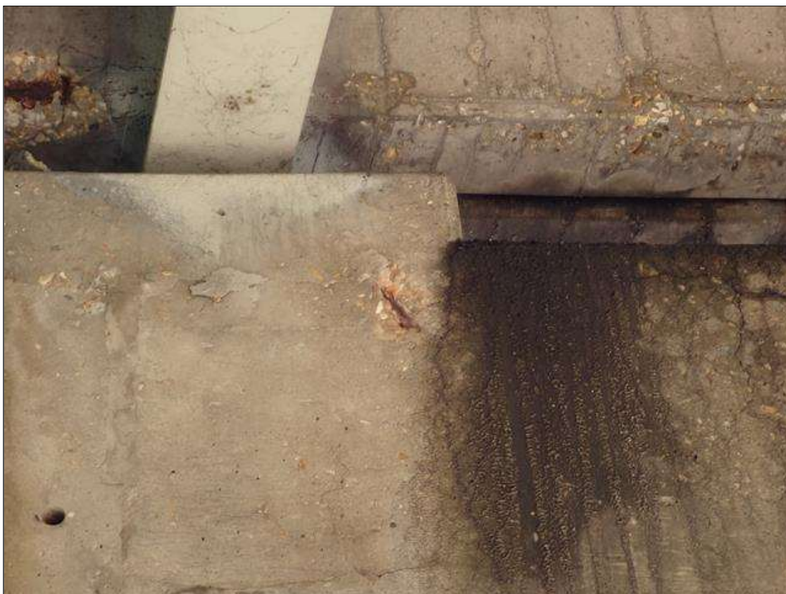
Bent 3 Cap 1: 5 INCH DIAMETER X 1/2 INCH SPALL WITH EXPOSED REBAR NORTH FACE UNDER BEAM 2
