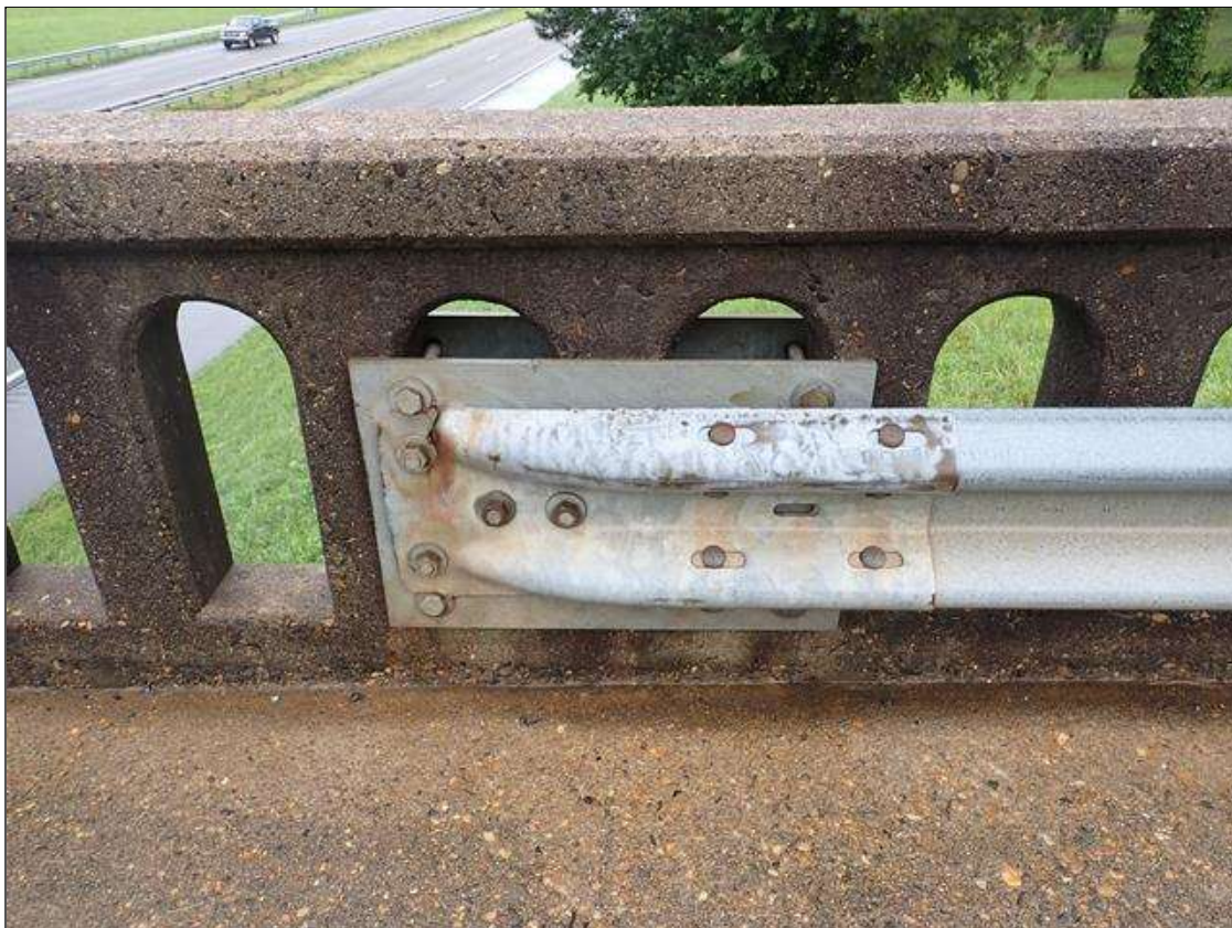
(PAR) northwest guardrail attachment, improper lap
