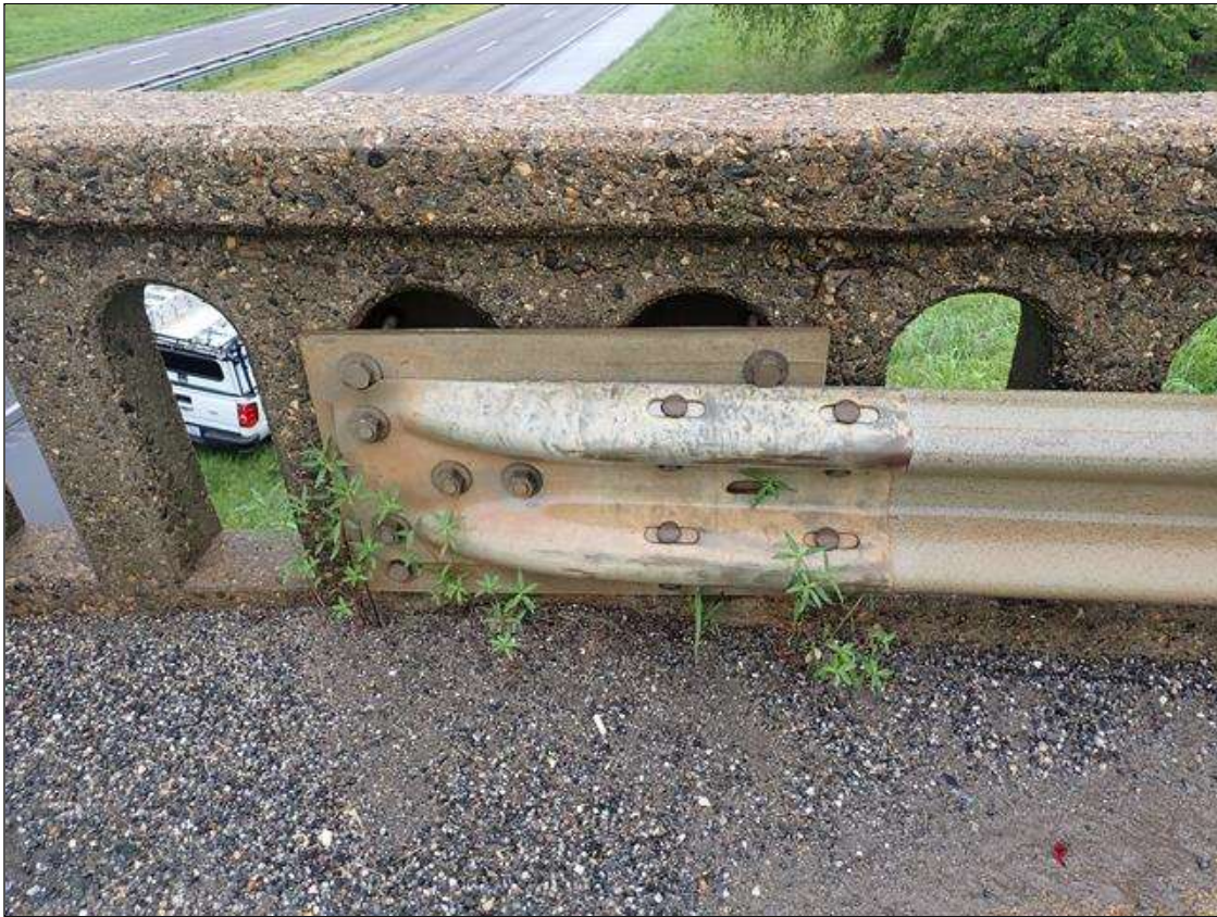
(PAR) southeast guardrail attachment, improper lap
