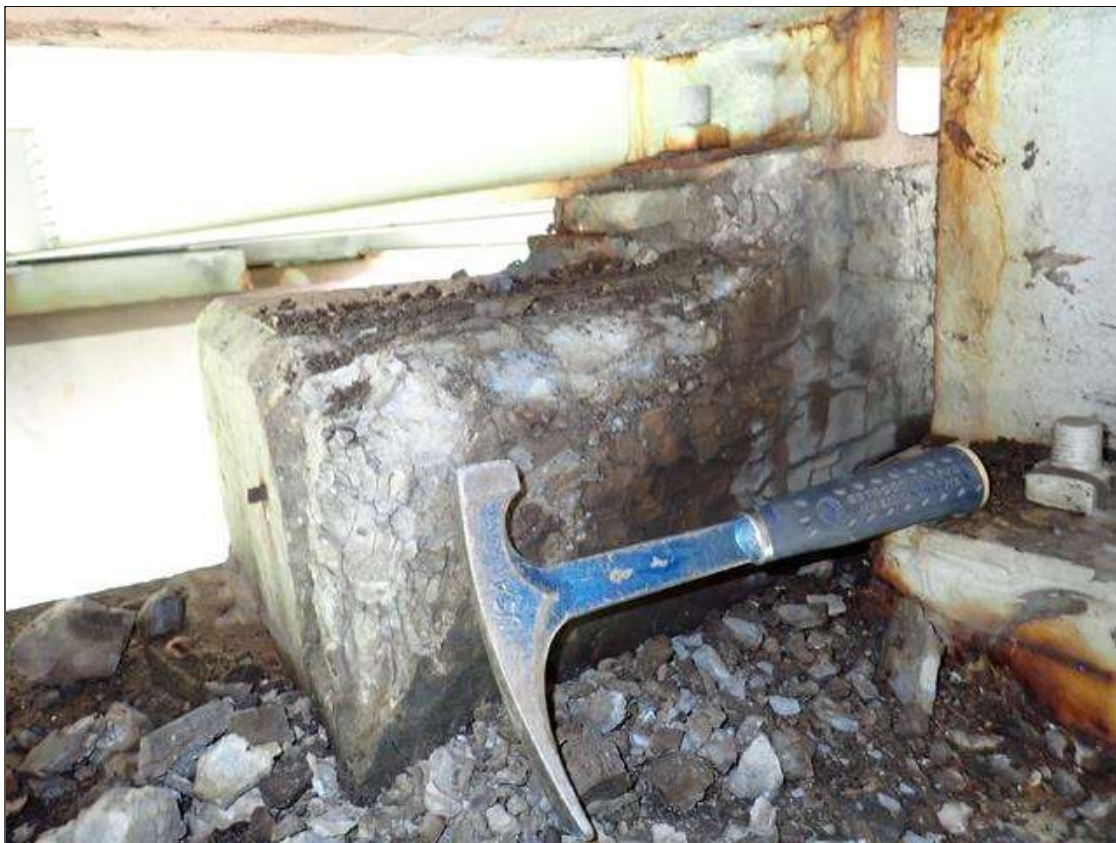
Bent 1 Cap 1: beam 3 cap step up, north face, failed patch (3 foot x 8 inch x 1 inch deep)
