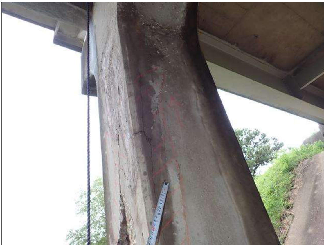
Bent 1 Pile 3: west face, delamination (1 foot x 6.5 foot) with cracks (up to 1/8 inch)
