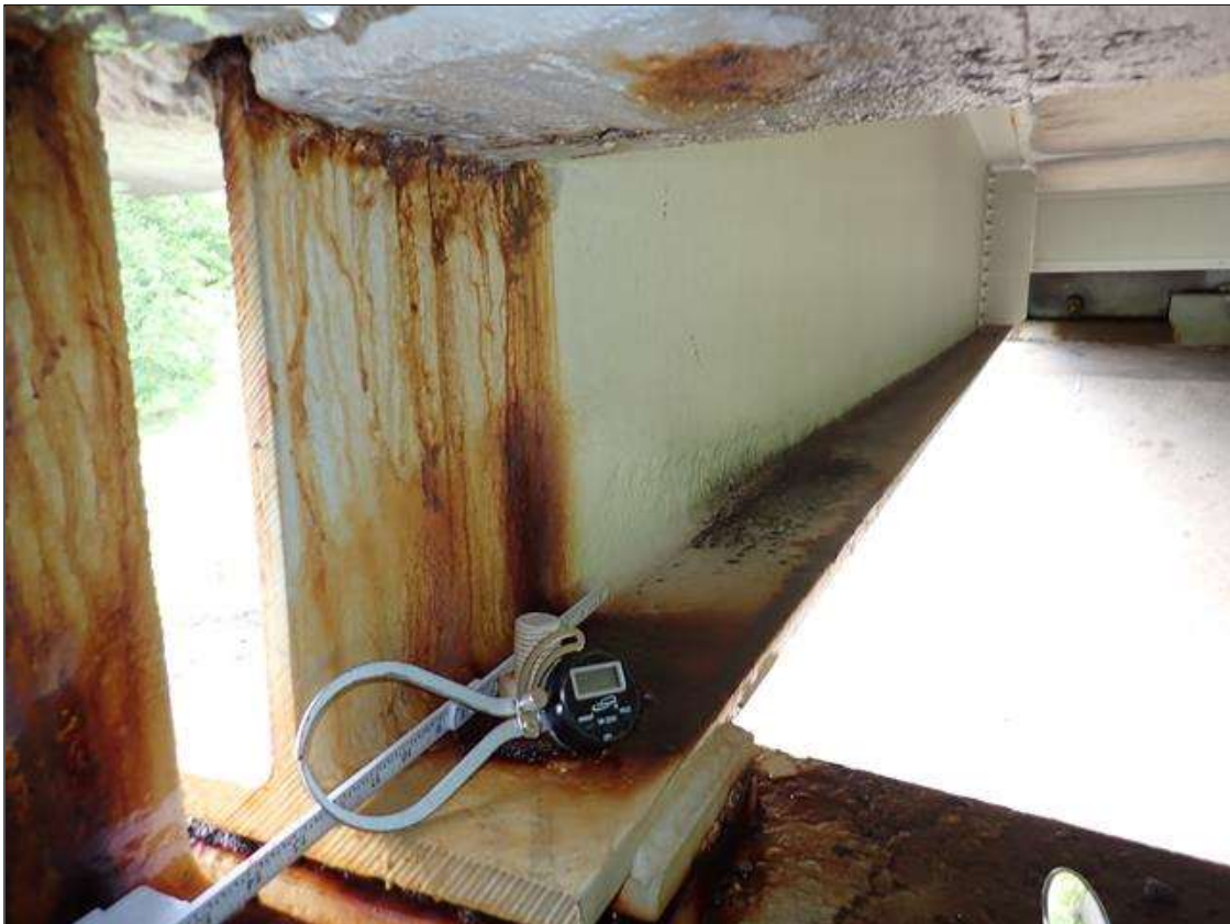
Span 1 Beam 5: (PAR) at bent 1, painted over section loss/pitting: upper web (7/16 inch average remaining x 11 inch x 8 inch); lower web (1/2 inch average remaining x 8 foot x 2 inch) with corrosion reactivating
