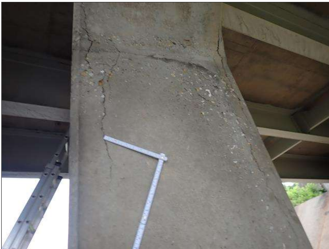
Bent 1 Pile 2: below cap, all corners, delaminations (1 foot x 3 foot) with cracks (up to 1/8 inch)
