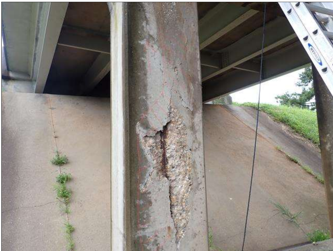
Bent 1 Pile 3: (PAR) north face, spall/delamination (2 foot x full height x 2 inch deep) with exposed rusted rebar (approximately 25 percent loss)
