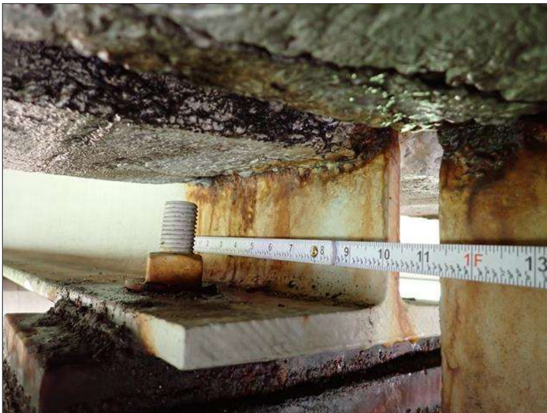
Span 1 Beam 4: at bent 1, corrosion with section loss/pitting: web adjacent to end diaphragm (7/16 inch average remaining x 10 inch x 2 inch)
