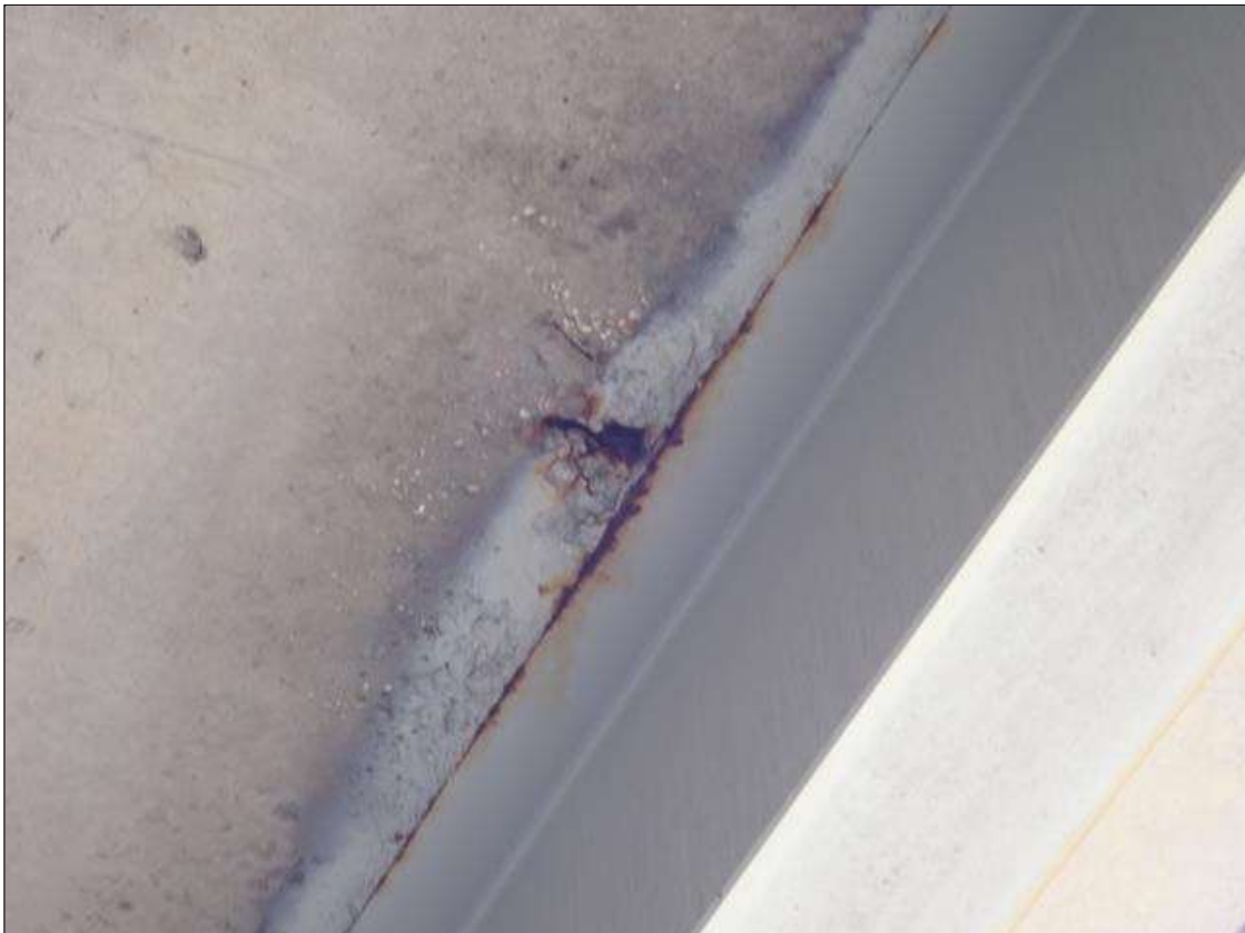
Span 2 Deck: (PAR) 2 FOOT X 1 FOOT X 3/4 INCH DEEP SPALL WITH EXPOSED REBAR BAY 1 ADJACENT TO BEAM 1 15 FOOT FROM BENT 2
