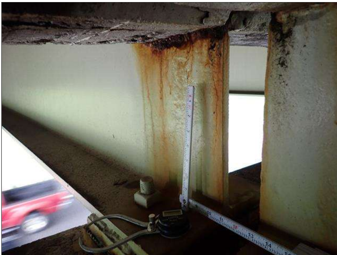
Span 3 Beam 2: (PAR) at bent 2, painted over section loss/pitting: web adjacent to end diaphragm (3/8 inch average remaining x 9 inch x 2 inch)
