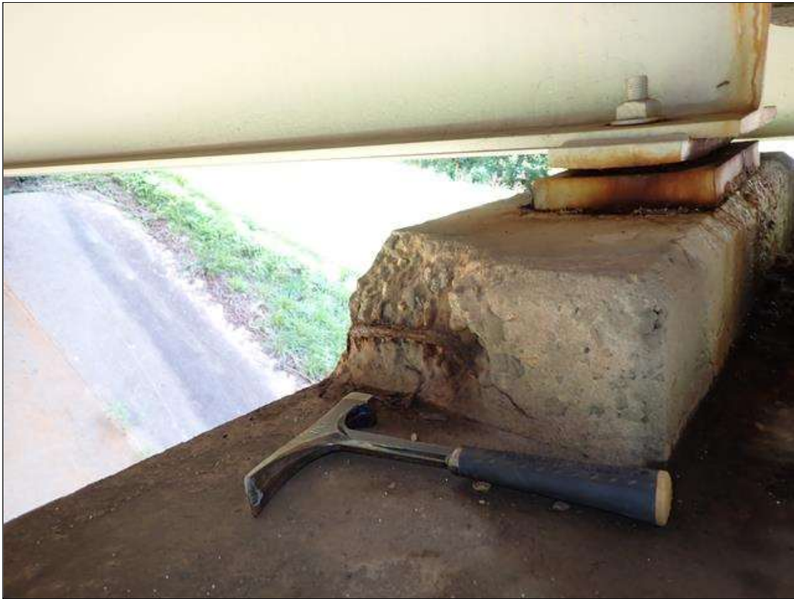
Bent 3 Cap 1: (PAR) 16 INCH X FULL HEIGHT X 2 INCH DEEP SPALL WITH EXPOSED REINFORCING WITH APPROXIMATELY 25 PERCENT LOSS, WEST FACE, IN BEAM 4 PEDESTAL.
