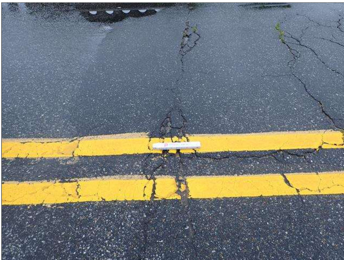
Span 1 Wearing Surface: over end bent 1, transverse cracks (up to 1/18 inch x full roadway width) with edge spalling (2 foot x 6 inch x 1.5 inch deep)
