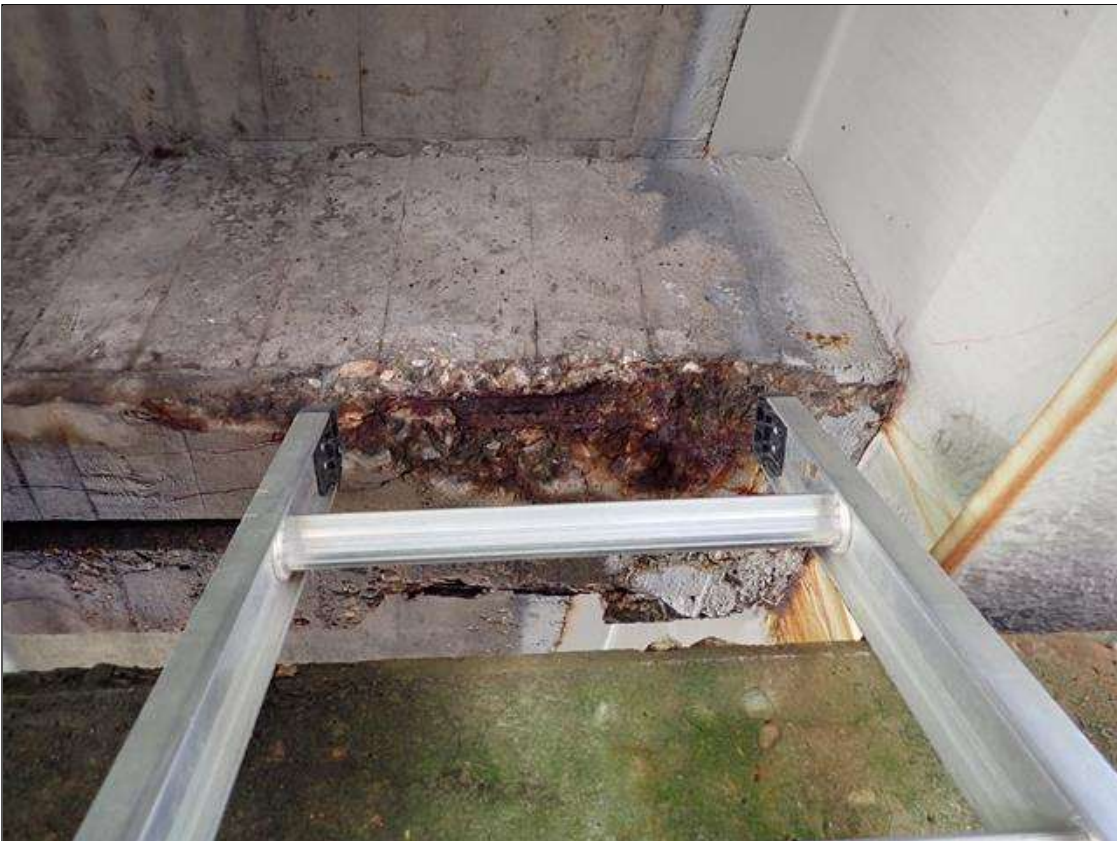
Span 2 Deck: (PAR) bays 1 and 4 end diaphragm over bent 2, spalls/delaminations (3 foot x 8 inch x 1 inch deep) with exposed rusted rebar (approximately 25 percent loss)
