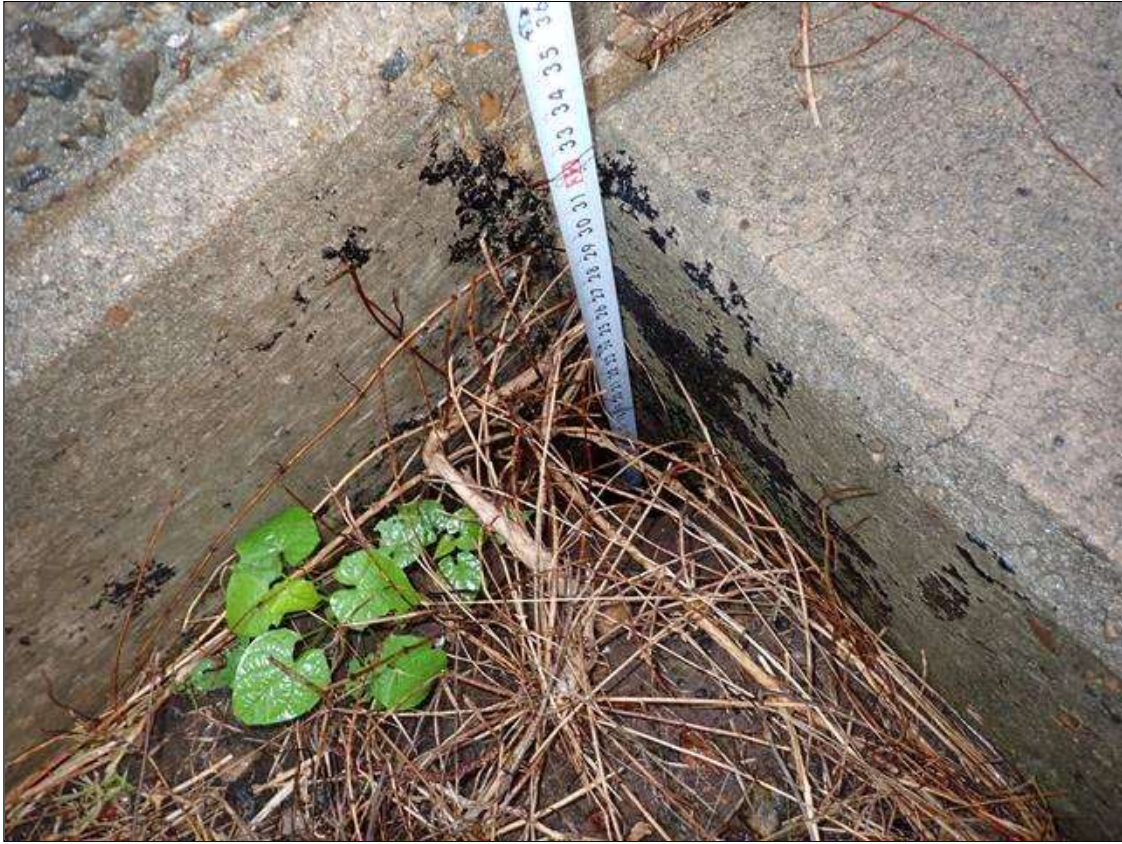
behind northwest wingwall, erosion hole (5 inch diameter x 2 foot deep)
