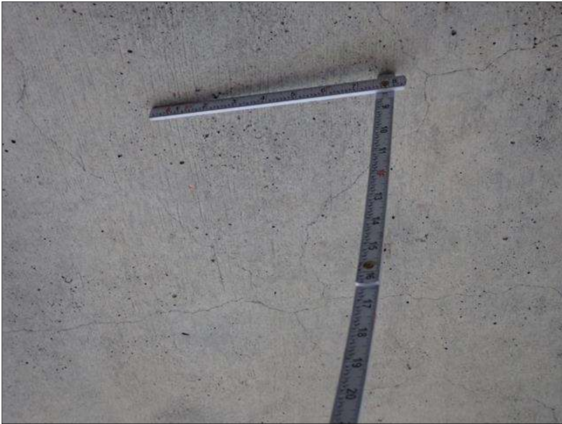
Span 1 Deck: throughout underside of deck, transverse cracks (up to 1/64 inch x full width) and map cracks (hairline) at random
