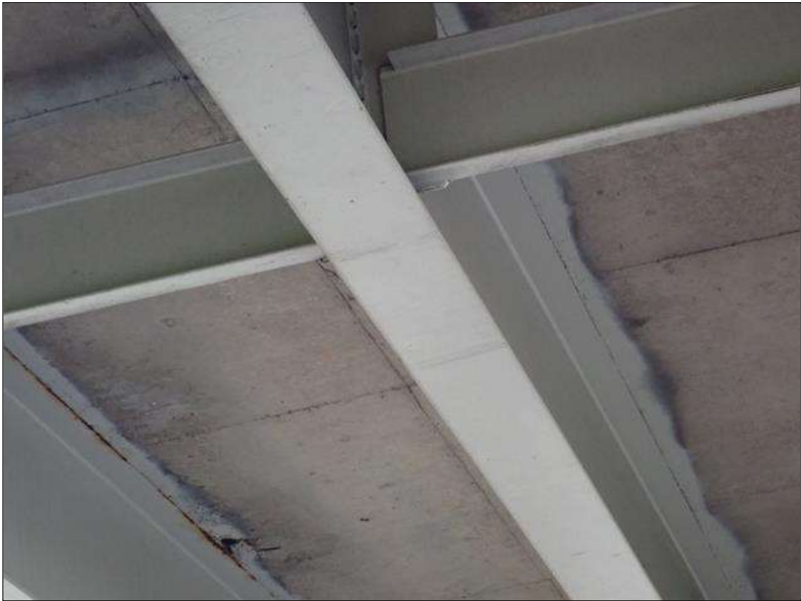
Span 2 Beam 2: SCATTERED SCRAPES TO BOTTOM FLANGE THROUGHOUT BEAM 2
