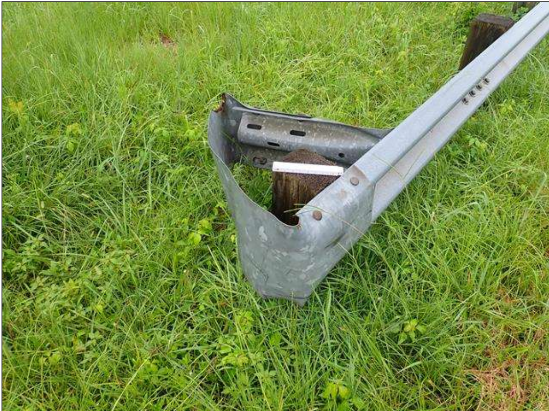
(PAR) northeast guardrail termination, impact damage
