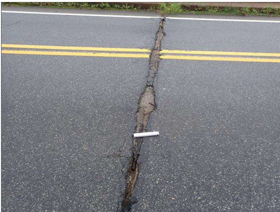
Span 2 Wearing Surface: (PAR) over bent 2, broken asphalt (full roadway width x 8 inch) with potholes (up to 10 foot x 9 inch x full depth)
