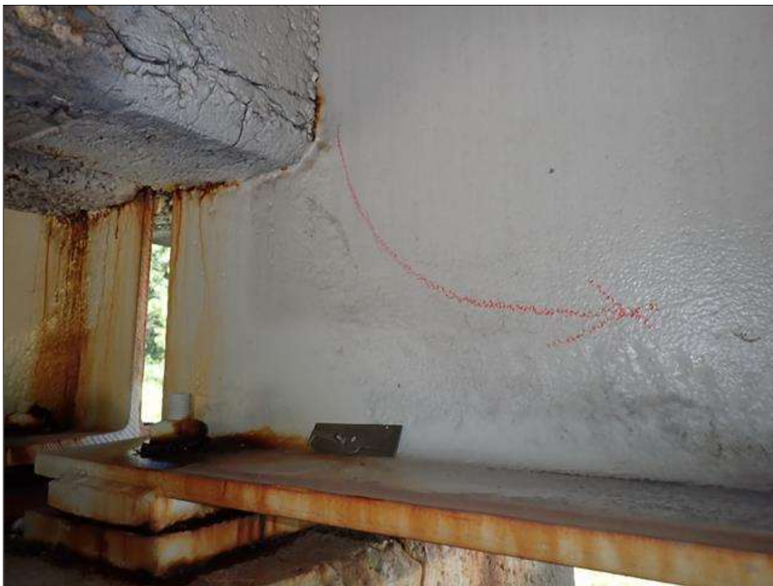
Span 3 Beam 5: at bent 3, painted over pitting/section loss: bottom flange (0.75 inch average remaining x 1 foot); bottom flange 1 foot from bearing, painted over pitting (up to 1/16 inch deep x 10 foot); web, painted over pitting (up to 1/8 inch deep x 10 foot x 12 inch)
