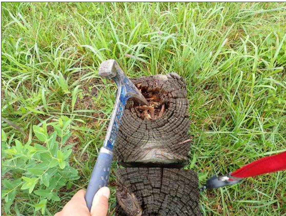
(PAR) southeast guardrail, timber posts 1-9, decay/section loss (up to full width x full height x full depth)
