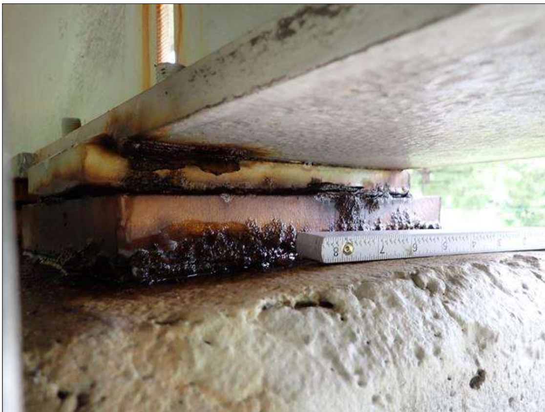
Span 2 Near Bearing 1: corrosion with section loss (up to 1/8 inch loss)
