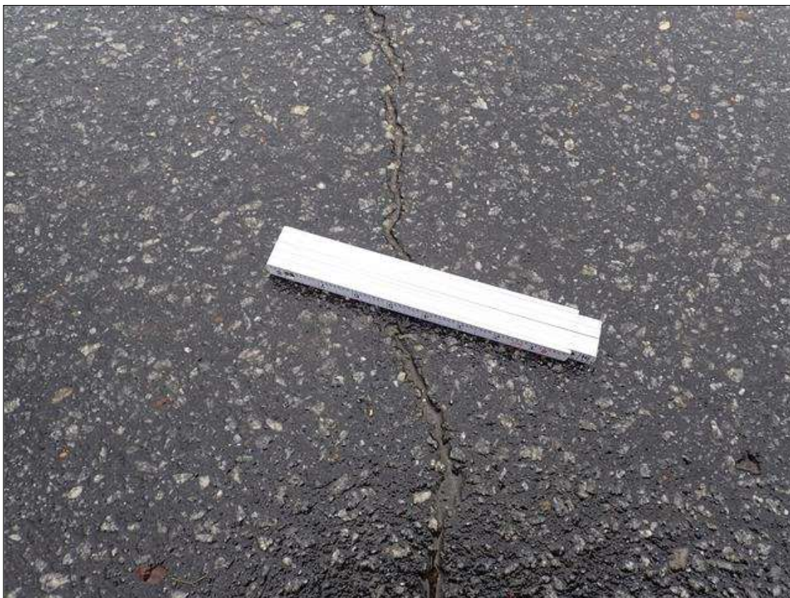
Span 1 Wearing Surface: throughout asphalt wearing surface, transverse and longitudinal cracks (up to 1/8 inch x 10 foot) at random
