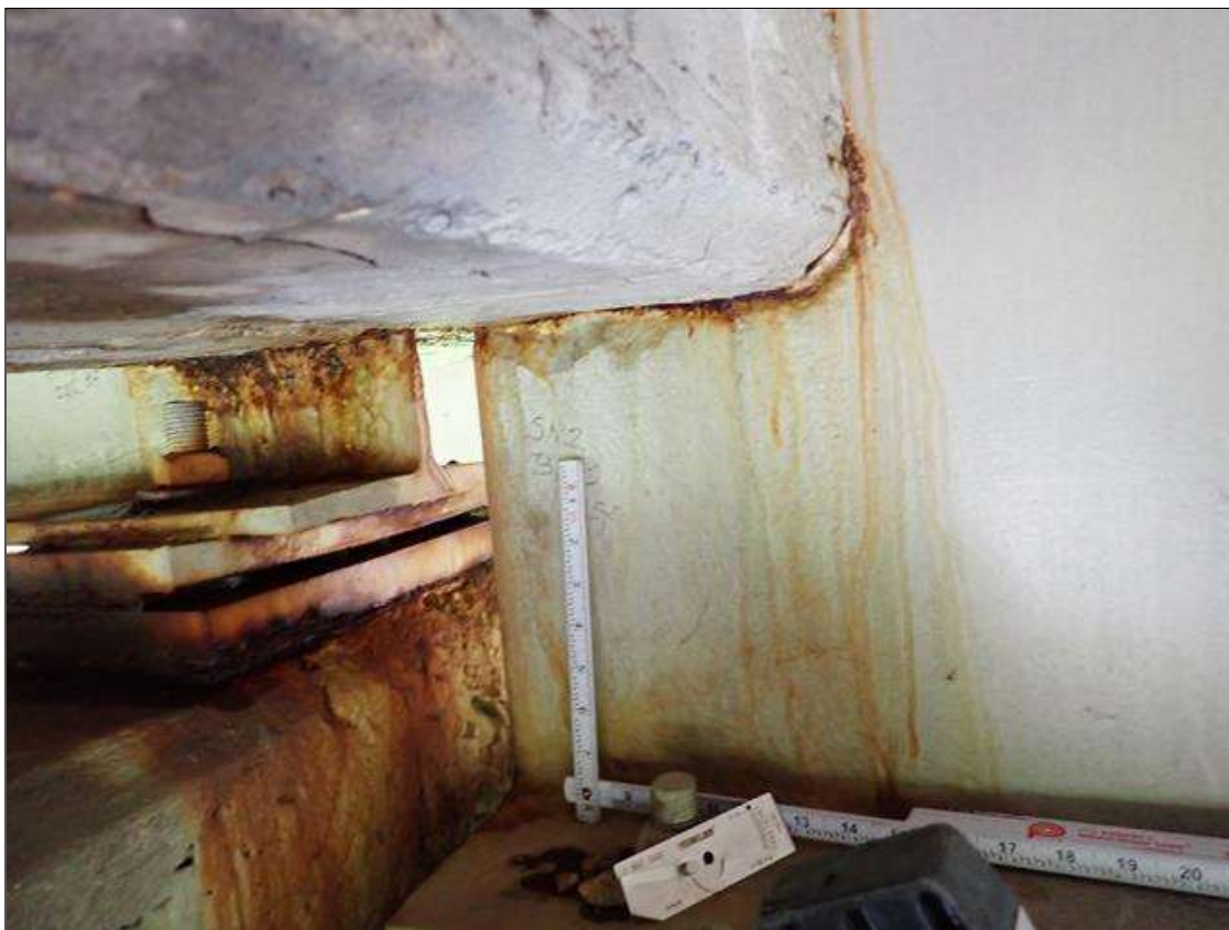
Span 2 Beam 2: (PAR) at bent 1, painted over section loss/pitting: web adjacent to end diaphragm (3/8 inch average remaining x 9 inch x 2 inch)
