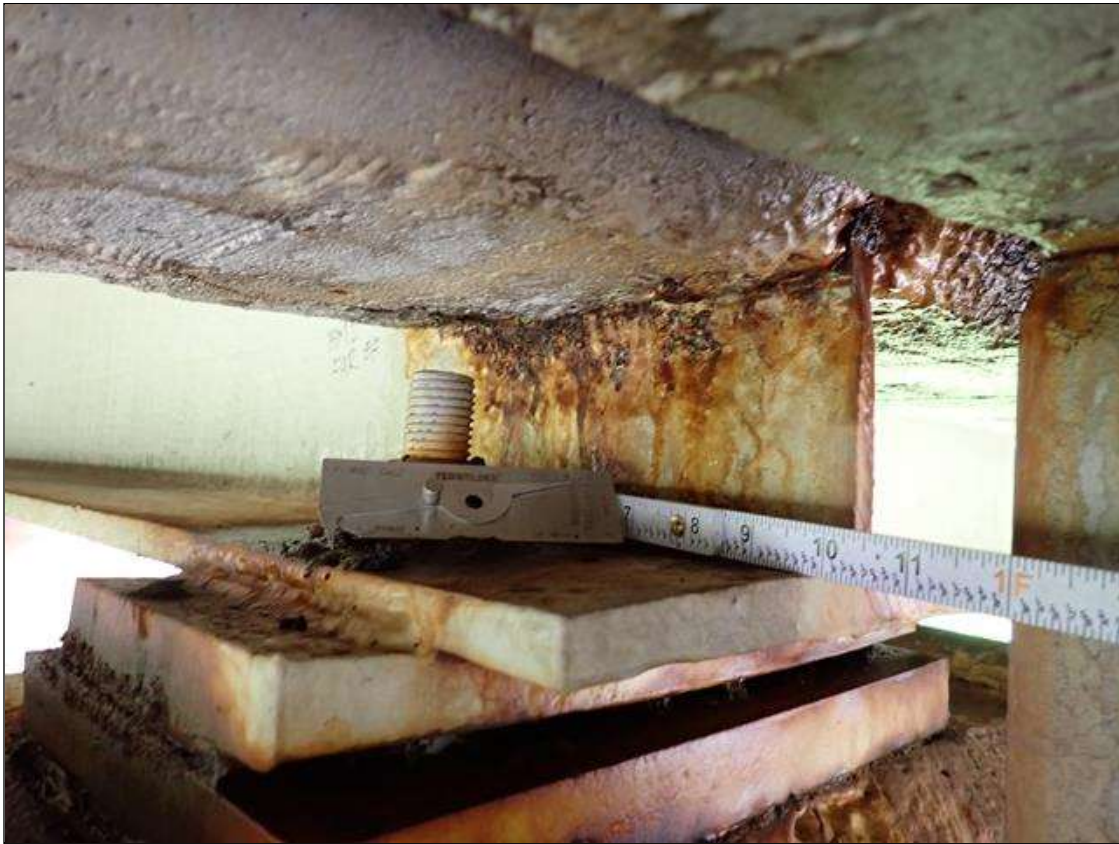
Span 1 Beam 2: (PAR) at bent 1, painted over section loss/pitting: web adjacent to end diaphragm (5/16 inch average remaining x 10 inch x 3.5 inch) with corrosion reactivating
