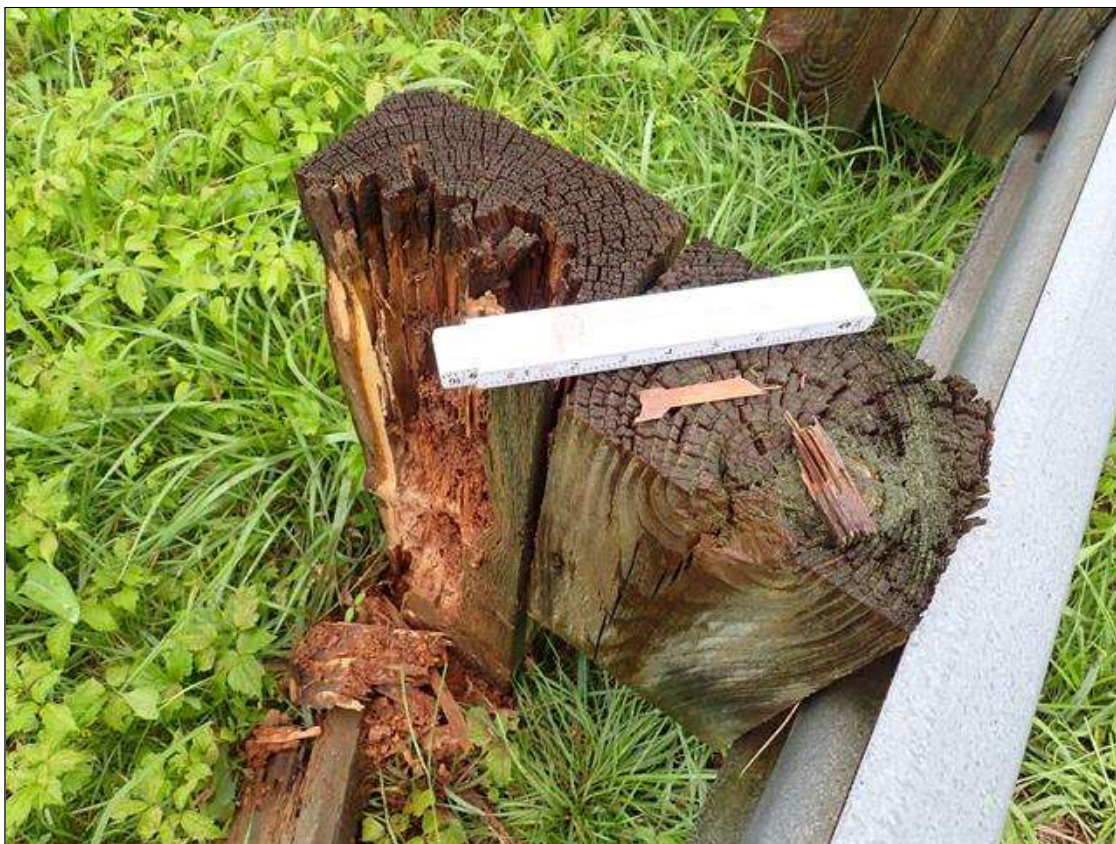
(PAR) northeast guardrail, 2nd, 4th and 6th timber posts, decay/section loss (up to full height x full width x full depth)
