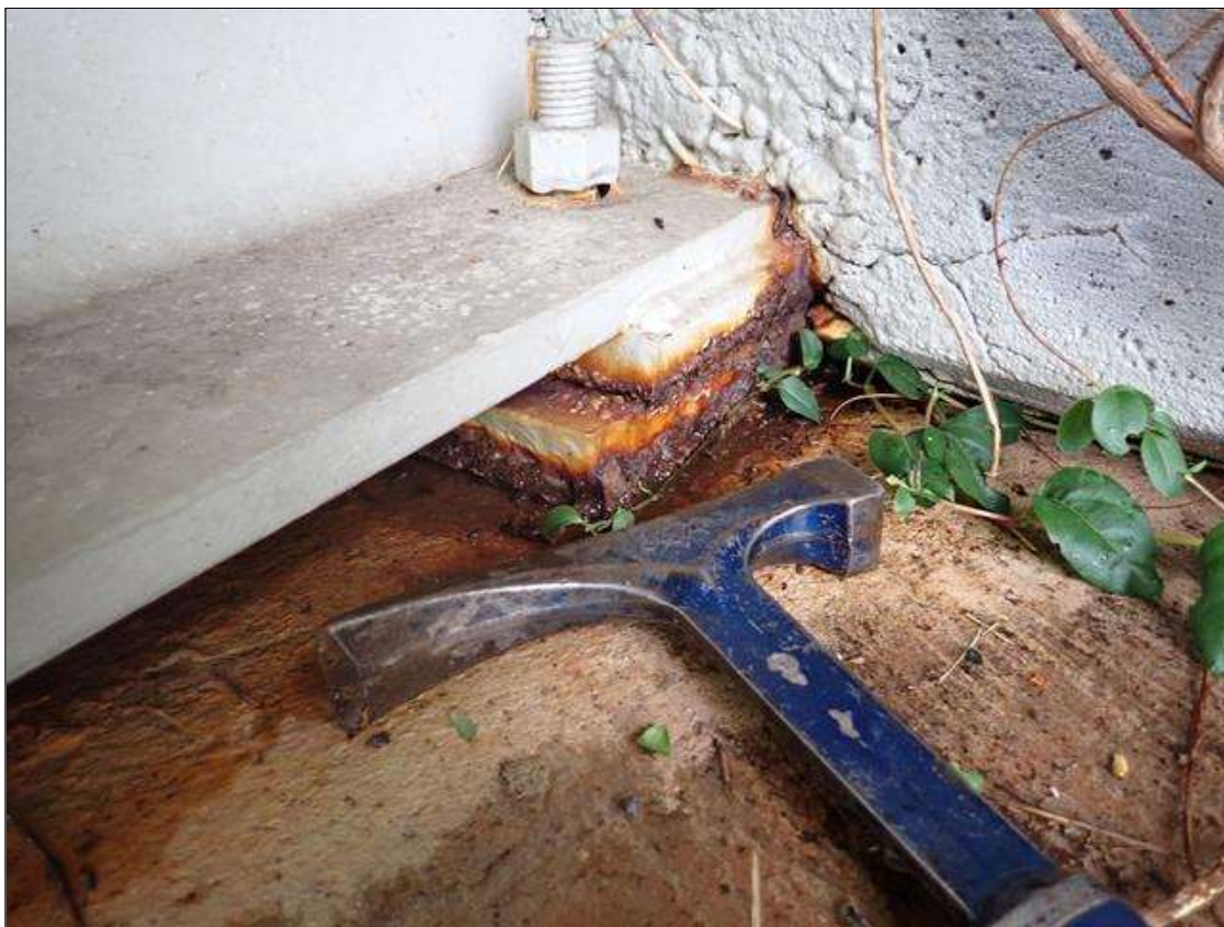
Span 4 Far Bearing 5: corrosion with section loss (up to 1/8 inch loss)
