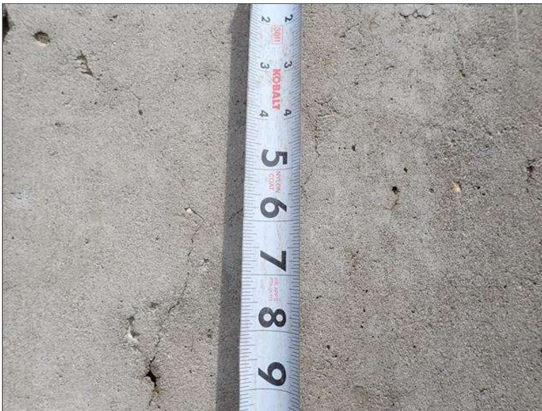
Bent 2 Pile 1: west face, map cracks (hairline) at random
