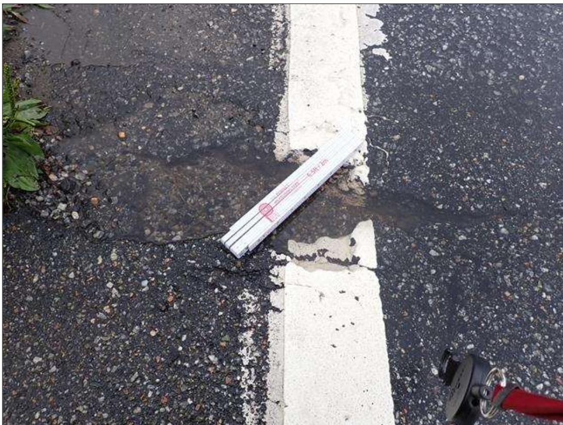
Span 1 Wearing Surface: over end bent 1, transverse cracks (up to 1/8 inch x full roadway width) with edge spalling (2 foot x 6 inch x 1.5 inch deep)
