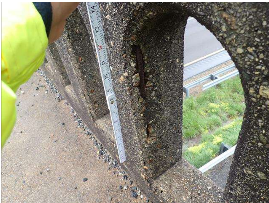
Span 2 Right Bridge Rail: UP TO 12 INCH X 3 INCH X 1/2 INCH DEEP SPALL WITH EXPOSED REBAR AT RANDOM THROUGHOUT
