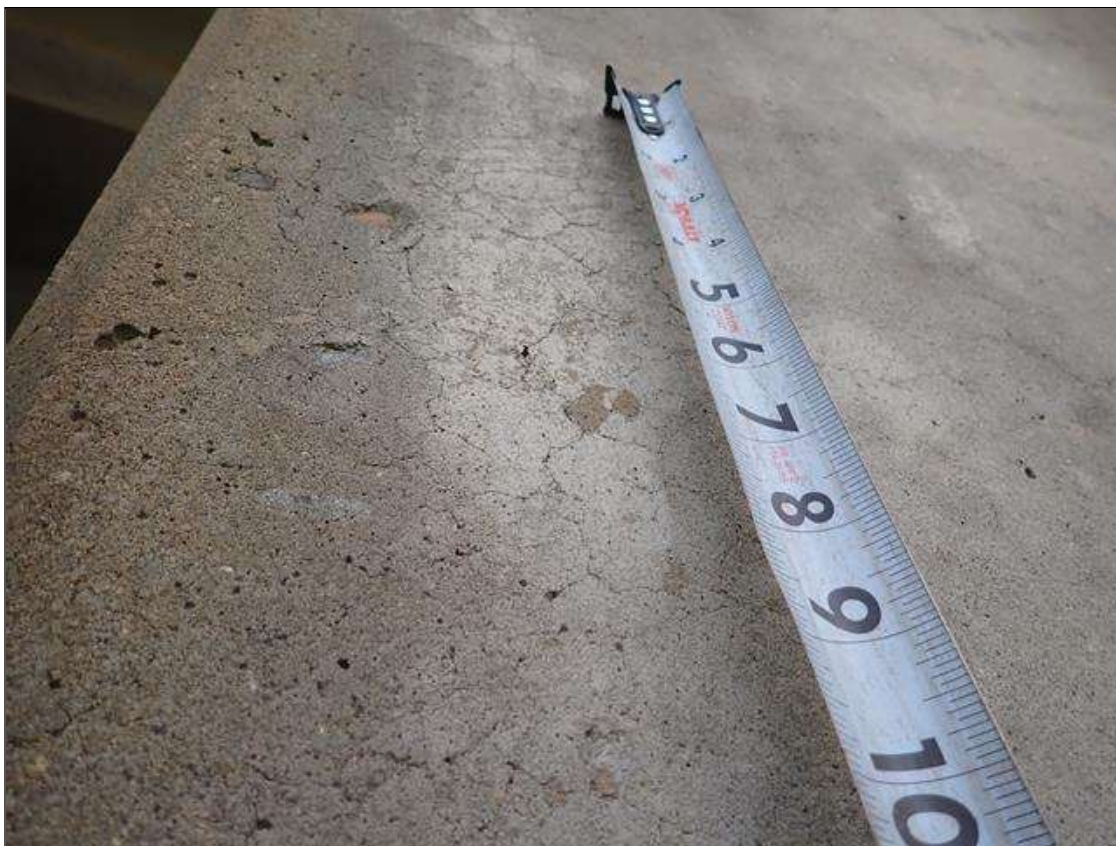
Bent 2 Pile 3: (PAR) along column, vertical cracks (up to 1/8 inch x 6.5 foot) some with efflorescence and rust stains and map cracks (hairline) at random
