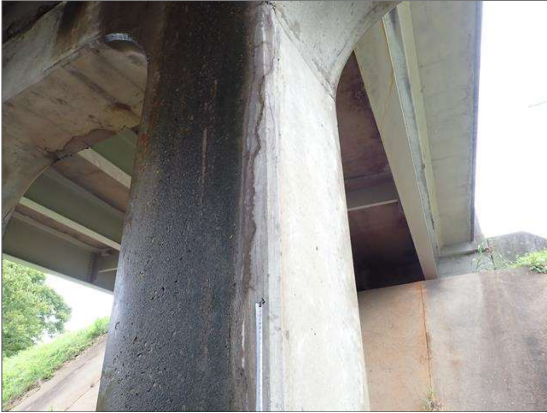
Bent 1 Pile 1: (PAR) NORTHWEST CORNER HAS A FAILED PATCHED AREA THAT IS CRACKED (UP TO 1/16 INCH) WITH RUST STAINS AND DELAMINATED. AREA ON NORTH FACE IS: 12 INCH WIDE, AREA ON WEST FACE IS: 10 INCH WIDE X 9 FOOT HIGH.
