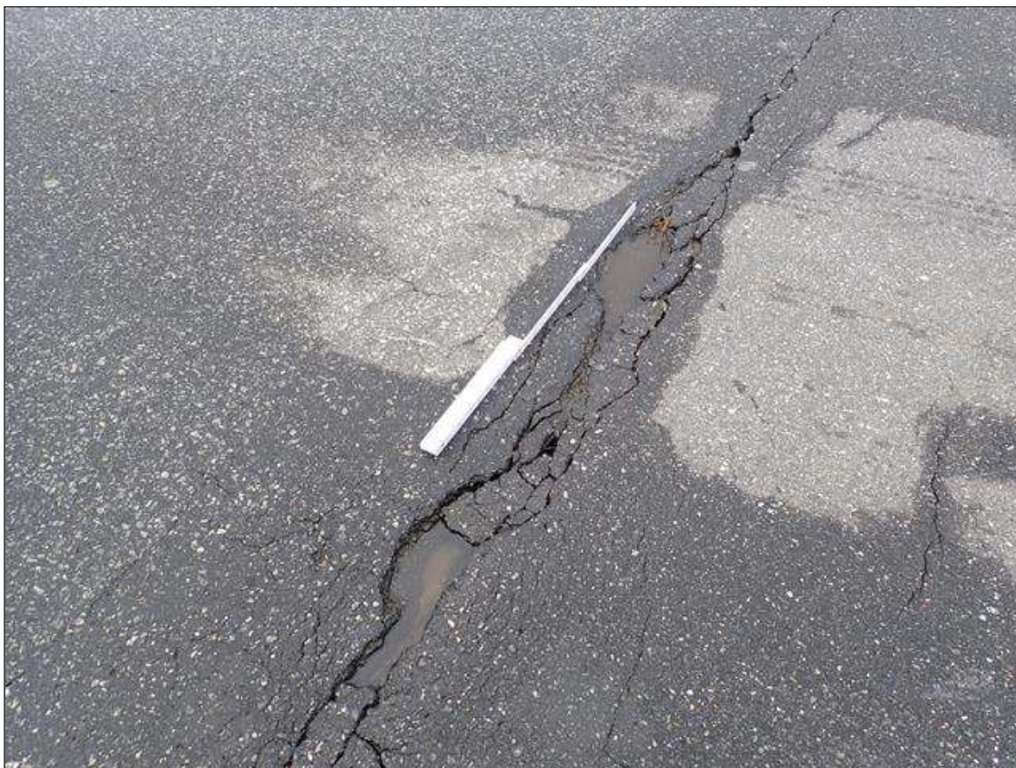
Span 4 Wearing Surface: over end bent 2, transverse cracks (up to 1/8 inch x full roadway width) with edge spalling (12 inch x 4 inch x 1 inch deep)
