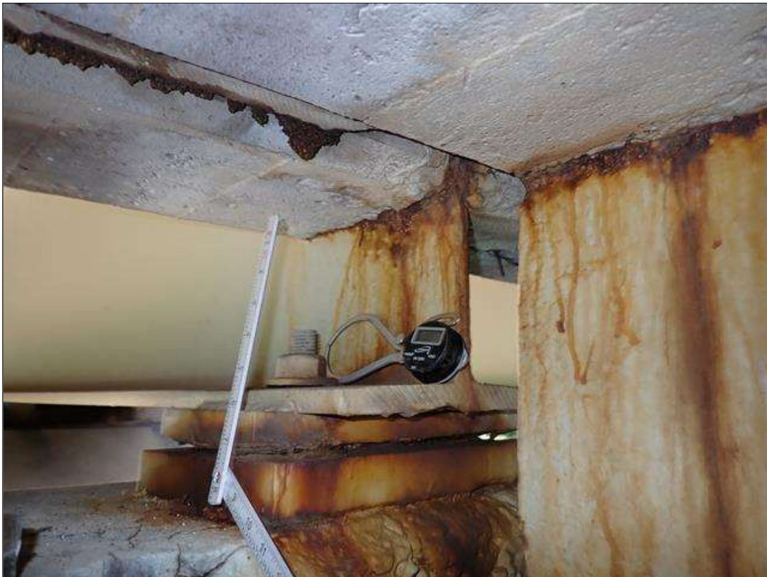
Span 4 Beam 3: (PAR) at bent 3, painted over section loss/pitting: web adjacent to end diaphragm (5/16 inch average remaining x 10 inch x 2 inch)
