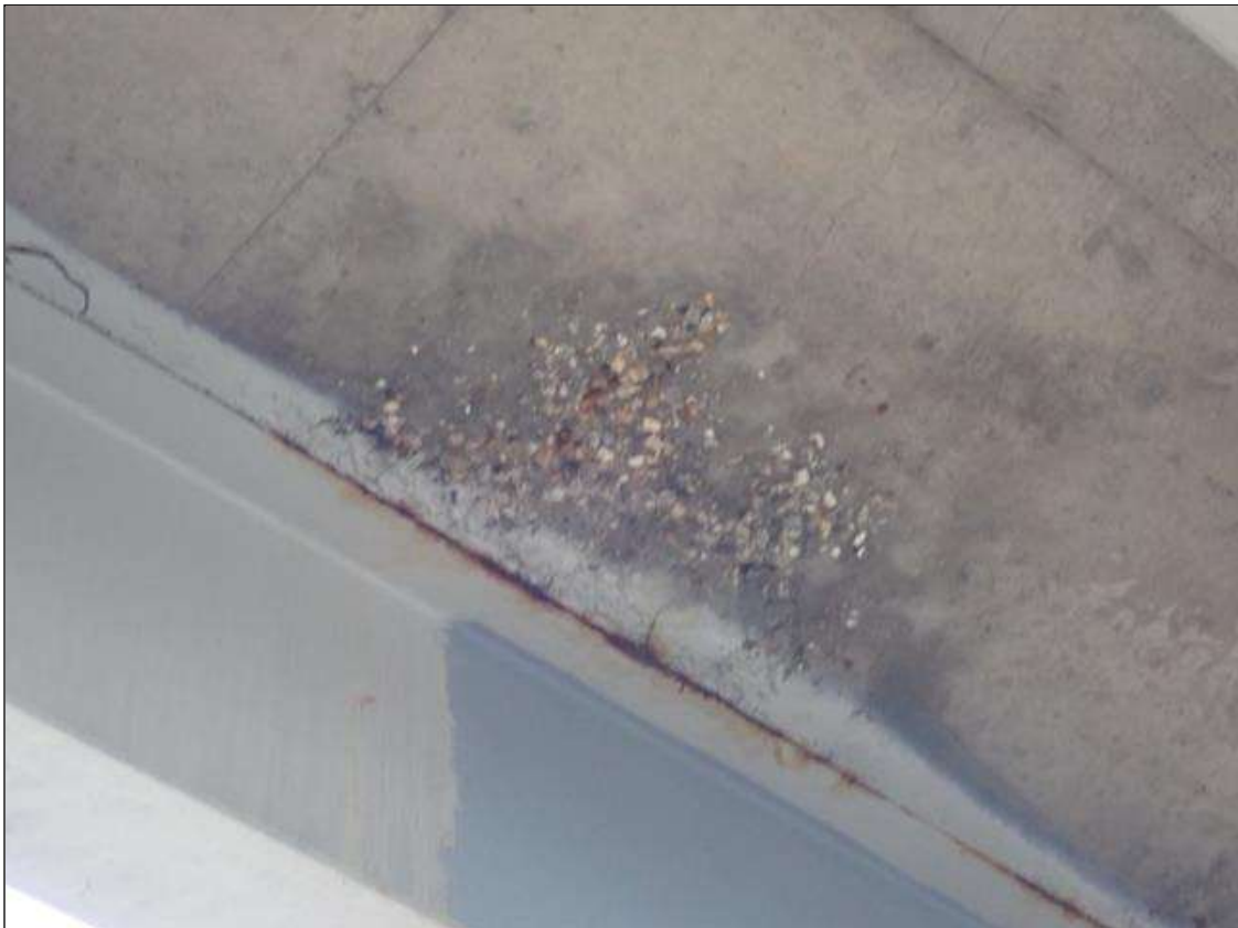
Span 2 Deck: MULTIPLE AREAS OF HONEYCOMBING IN BAYS 1 & 4 AT RANDOM THROUGHOUT.
