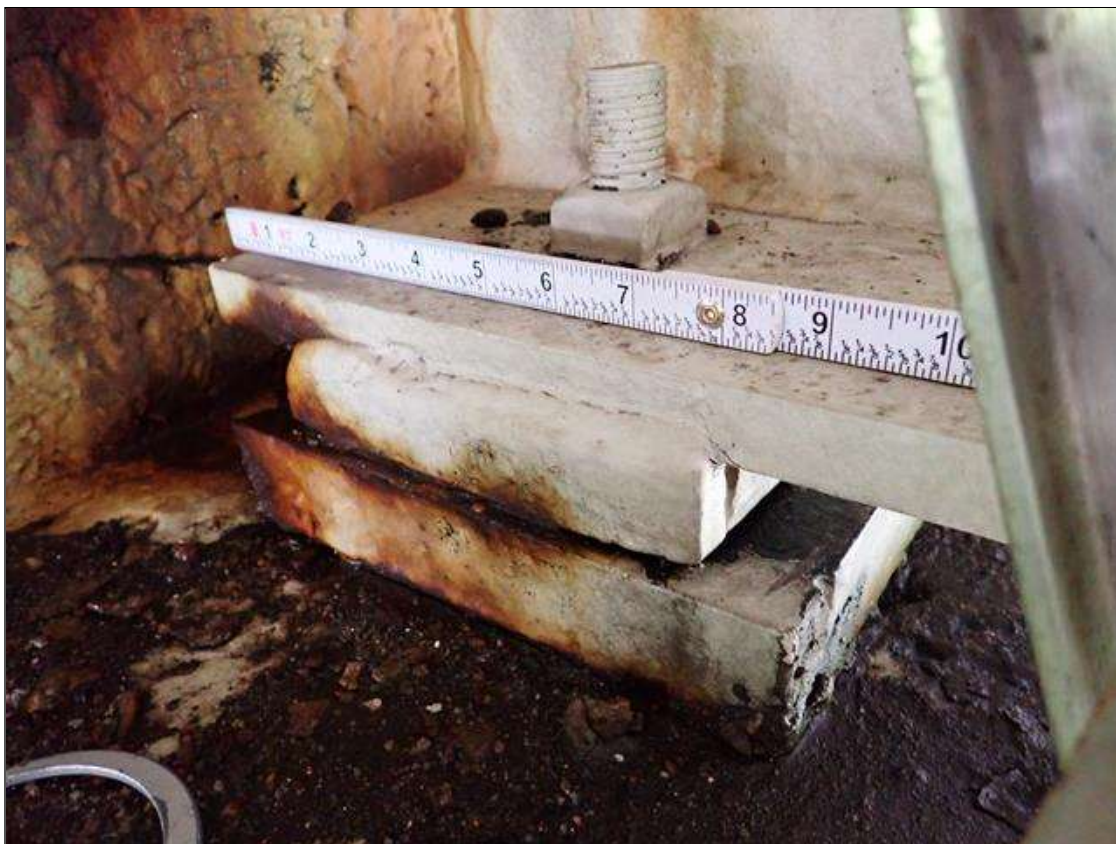
Span 2 Near Bearing 4: corrosion with section loss (up to 1/16 inch loss)
