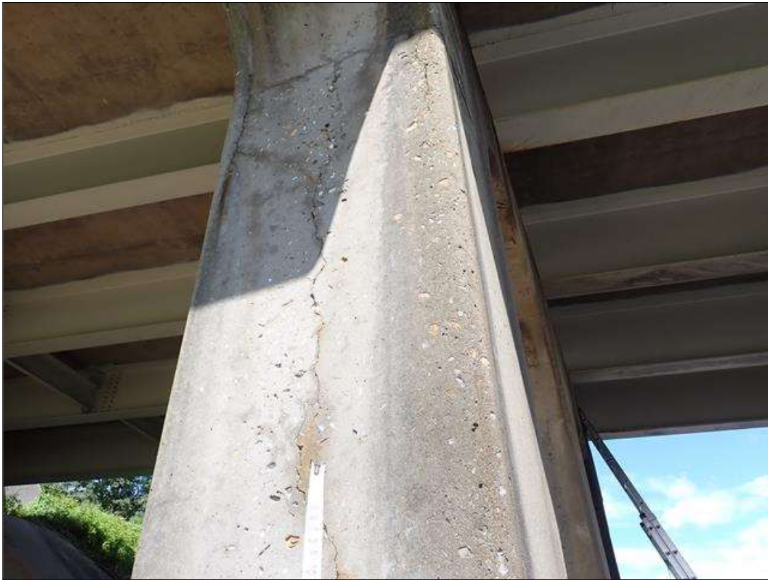
Bent 3 Pile 1: (PAR) WEST FACE HAS AN AREA THAT IS CRACKED (UP TO 1/16 INCH) AND DELAMINATED WITH SOME RUST STAINS VISIBLE AREA IS: 16 INCH X 10 FOOT.
