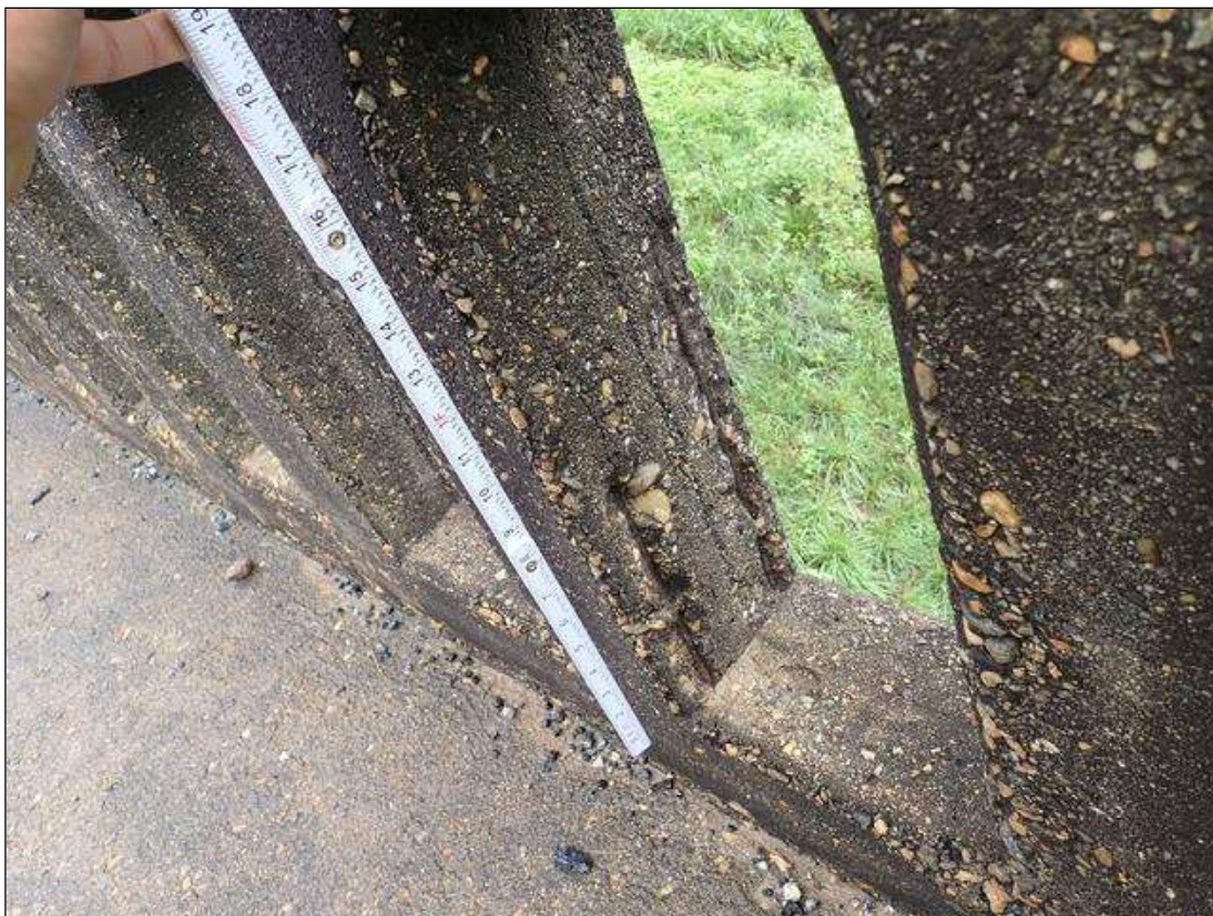
Span 4 Right Bridge Rail: UP TO 18 INCH X 3 INCH X 1/2 INCH DEEP SPALL WITH EXPOSED REBAR AT RANDOM THROUGHOUT
