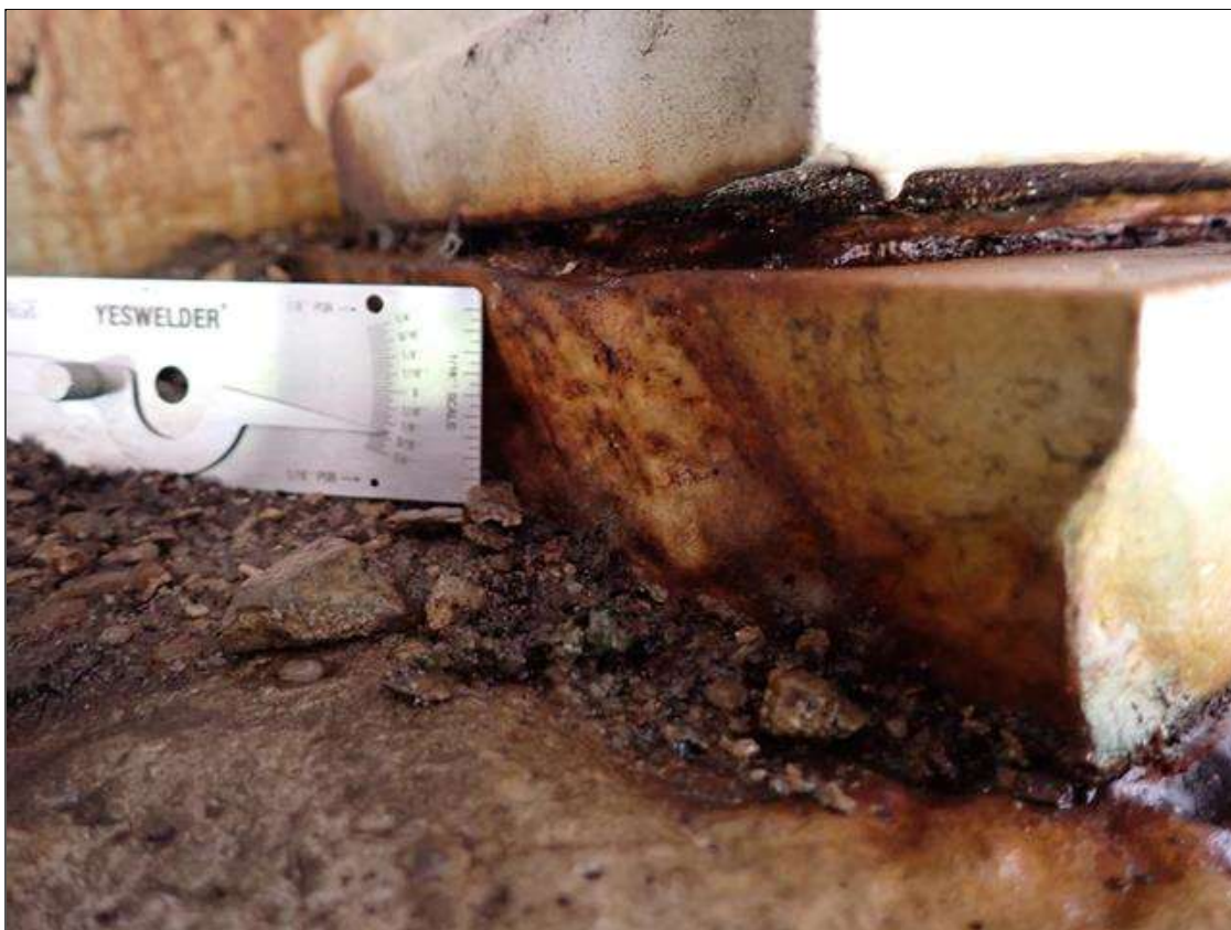
Span 2 Near Bearing 2: corrosion with section loss (up to 1/16 inch loss)
