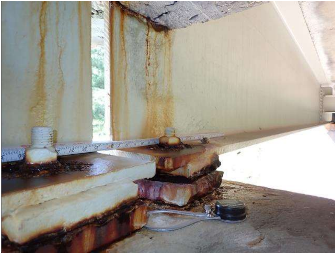
Span 4 Beam 1: at bent 3, painted over pitting: web (up to 1/8 inch deep x 2 foot x 12 inch); bottom flange (up to 1/16 inch deep x 2 foot)
