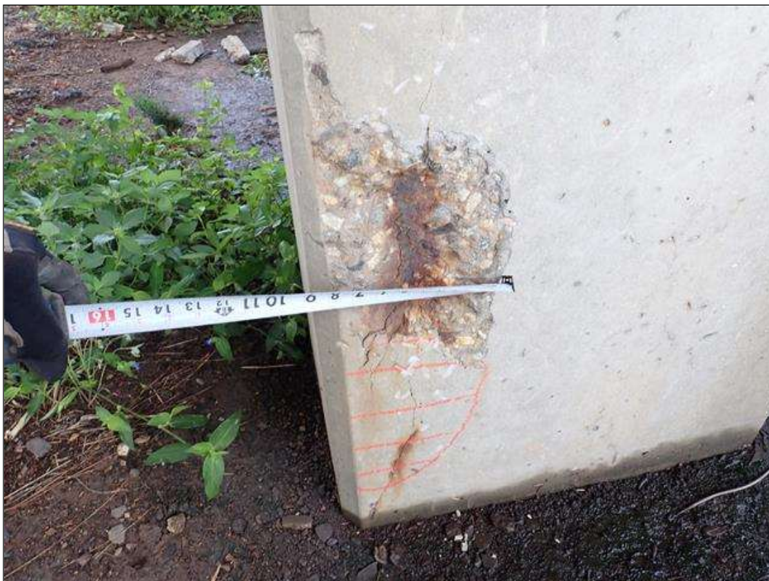
Bent 2 Pile 2: (PAR) west face at bottom, spall (2 foot x 8 inch x 1 inch deep) with exposed rusted rebar (approximately 25 percent loss)
