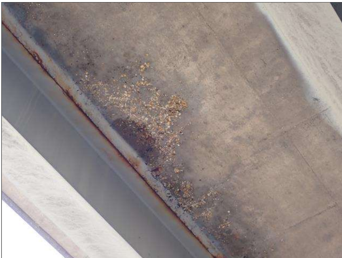
Span 3 Deck: MULTIPLE AREAS OF HONEYCOMBING IN BAYS 1 & 4 AT RANDOM THROUGHOUT.
