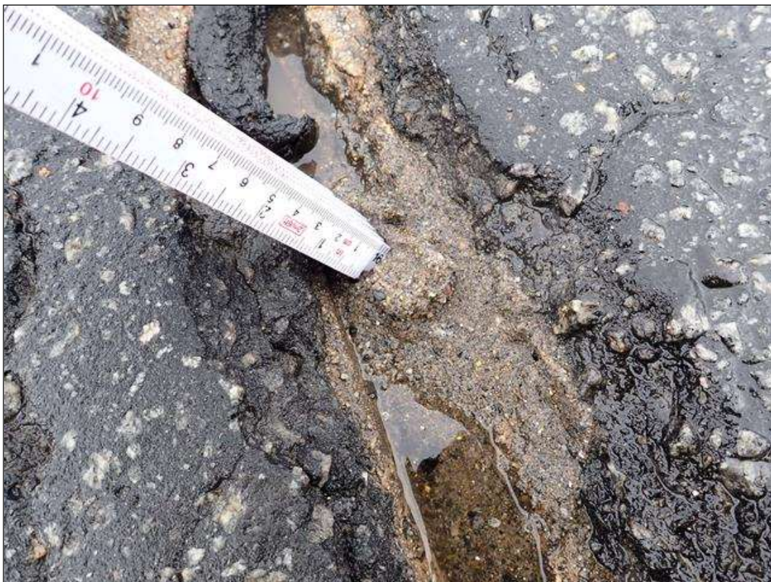
Span 2 Bent 1 Expansion Joint: at missing asphalt locations, debris accumulation (up to 32 inch) at random
