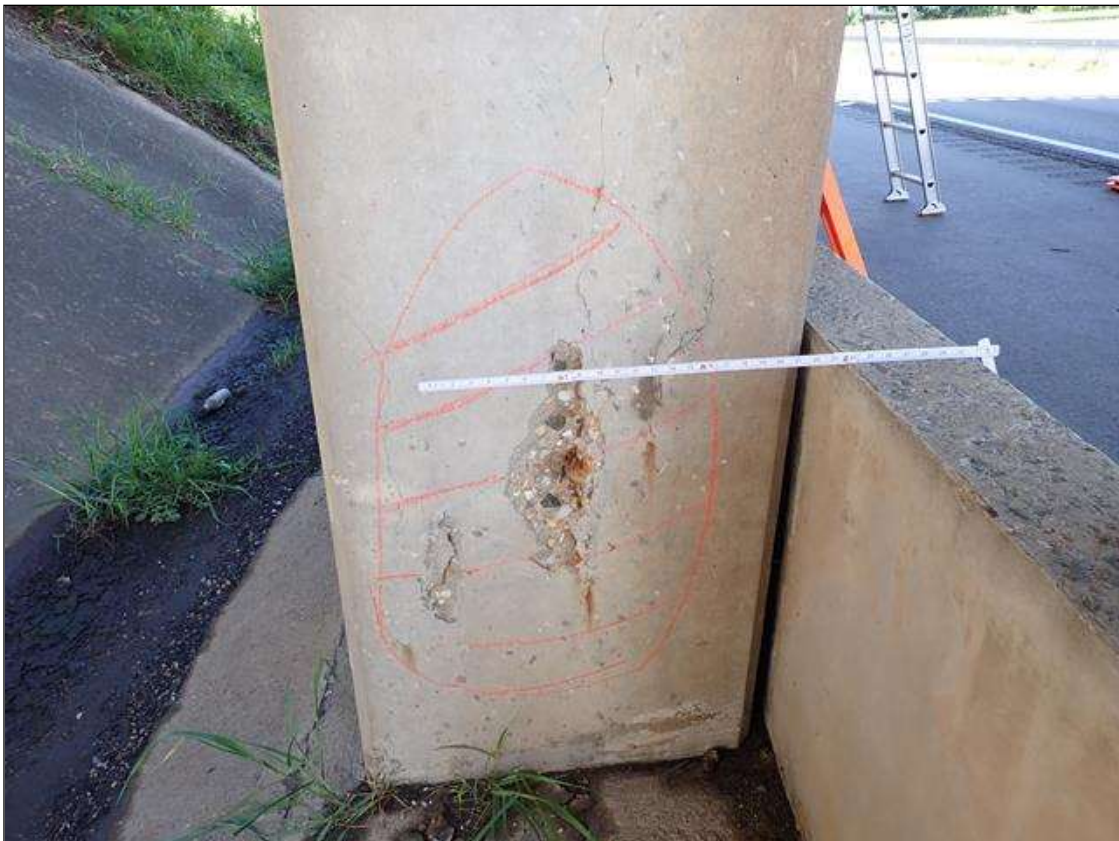
Bent 3 Pile 2: (PAR) west face at bottom, spall/delamination (3 foot x 21 inch x 1/2 inch) with exposed rusted rebar and cracks (up to 1/32 inch) with rust stains
