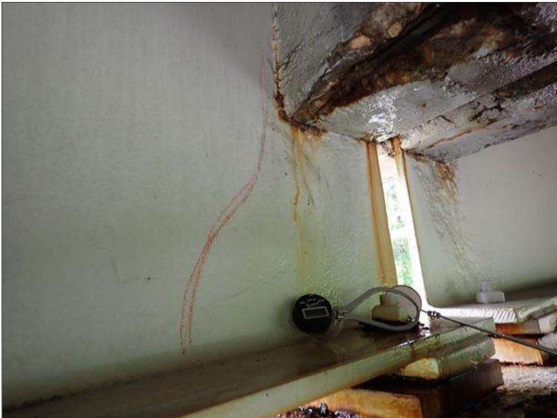
Span 2 Beam 1: at bent 2, painted over section loss/pitting: web adjacent to end diaphragm (1/2 inch average remaining x 16 inch x 13 inch); bottom flange, pitting (up to 1/16 inch deep x 16 inch) with corrosion reactivating
