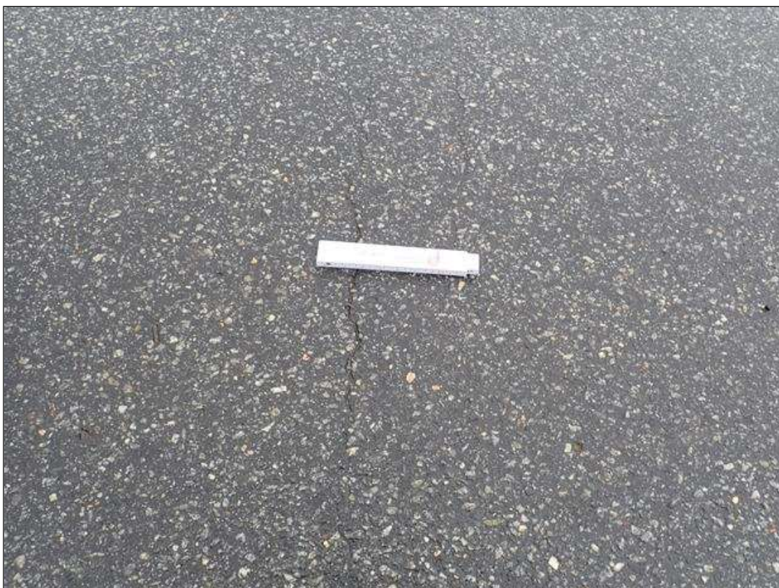
Span 2 Wearing Surface: throughout asphalt wearing surface, transverse and longitudinal cracks (up to 1/8 inch x 10 foot) at random
