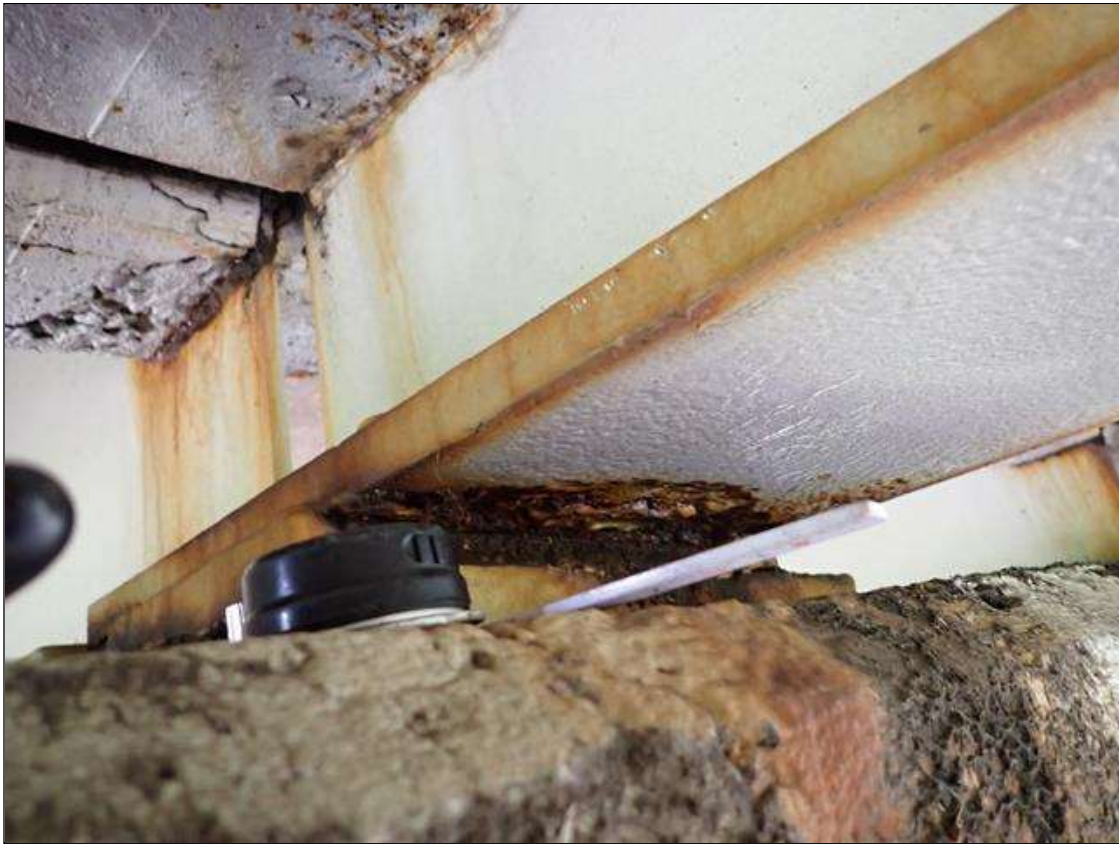
Span 2 Beam 2: (PAR) at bent 2, painted over section loss/pitting: bottom flange (0.73 inch average remaining x 3 inch); web adjacent to end diaphragm (3/8 inch average remaining x 10 inch x 6 inch)
