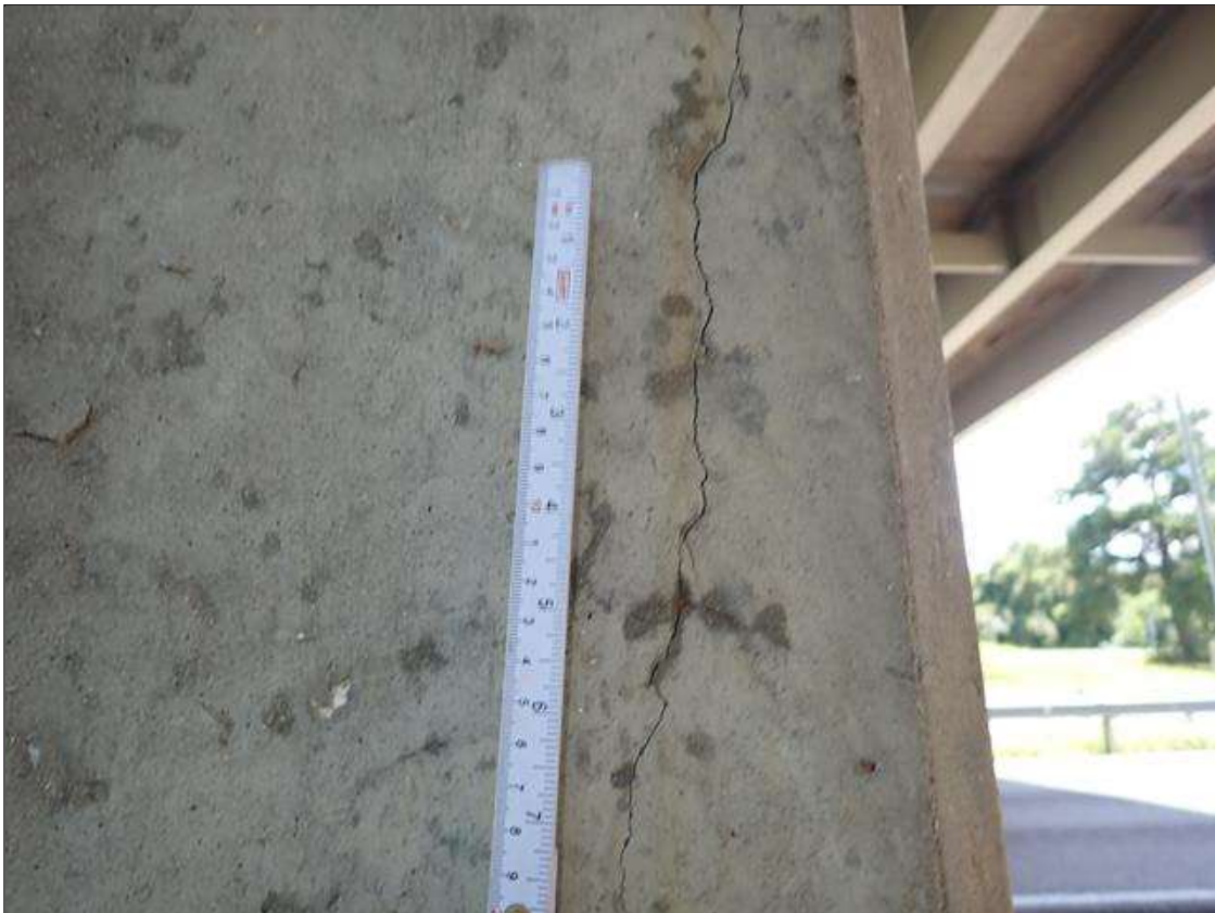
Bent 3 Pile 3: along column, vertical cracks (up to 1/32 inch x full height) and map cracks (hairline)
