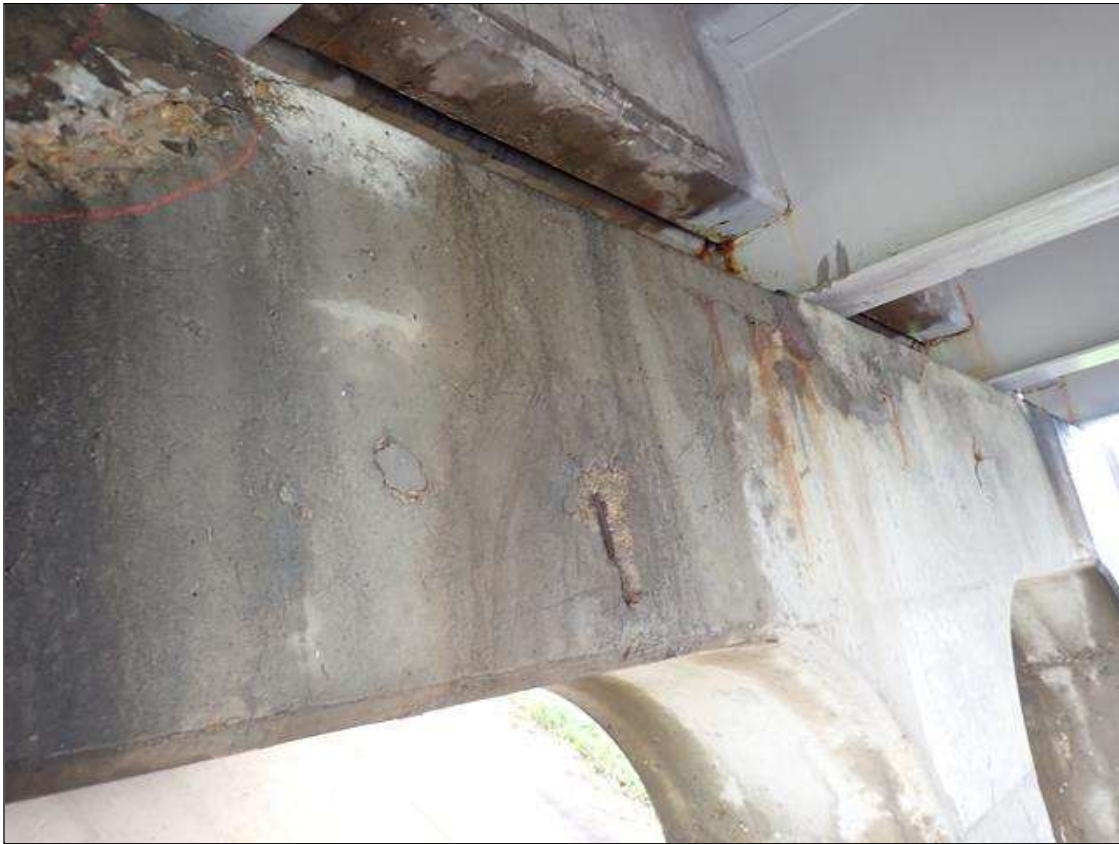
Bent 1 Cap 1: (PAR) south face between bays 2-4, multiple spalls/delaminations (5 foot x 16 inch x 1 inch deep) some with exposed rusted rebar (approximately 25 percent loss) and cracks (up to 1/16 inch) with rust stains
