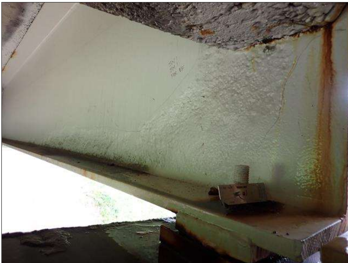
Span 1 Beam 1: at bent 1, painted over pitting: web (up to 1/8 inch deep x 11 foot x up to 16 inch) with corrosion reactivating
