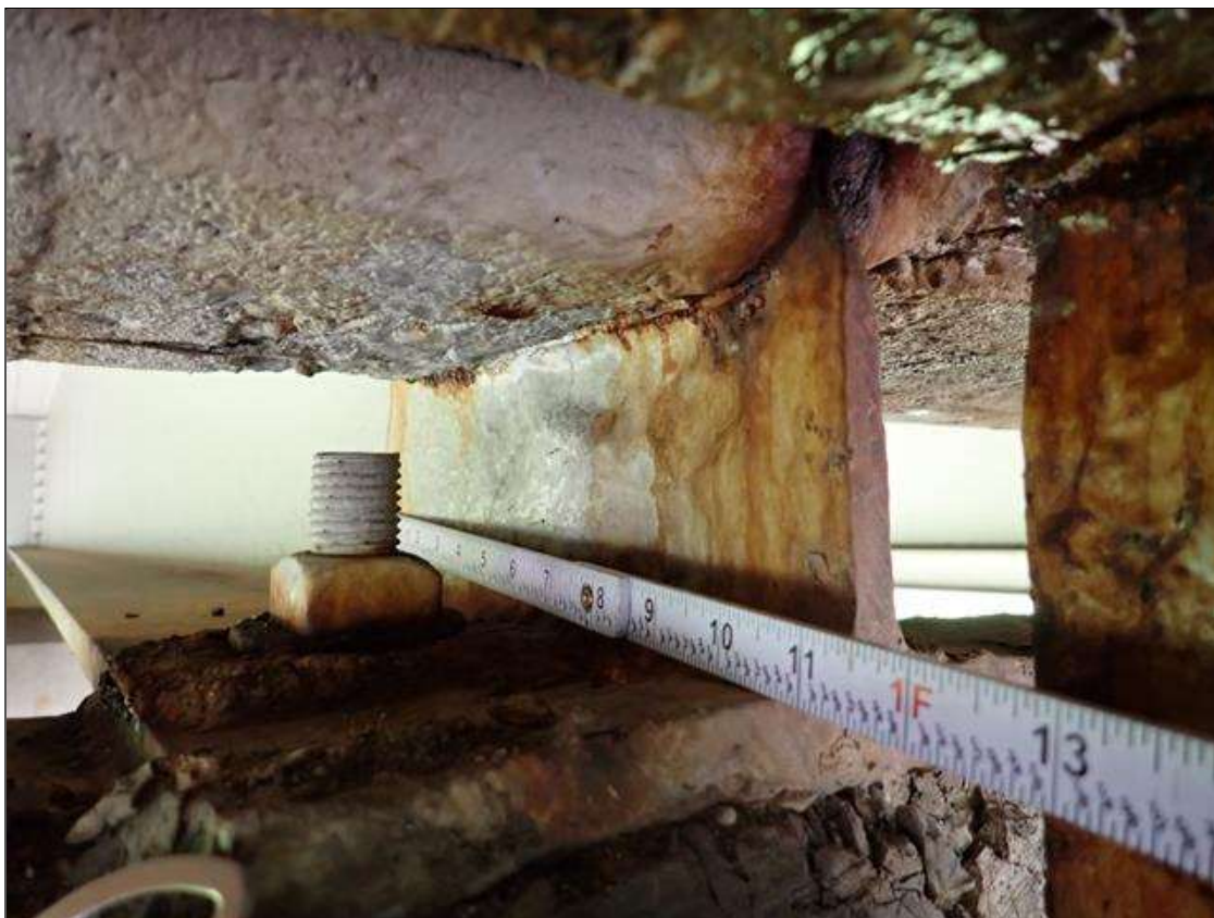
Span 1 Beam 3: (PAR) at bent 1, painted over section loss/pitting: web (1/4 inch average remaining x 11 inch x 3.5 inch)
