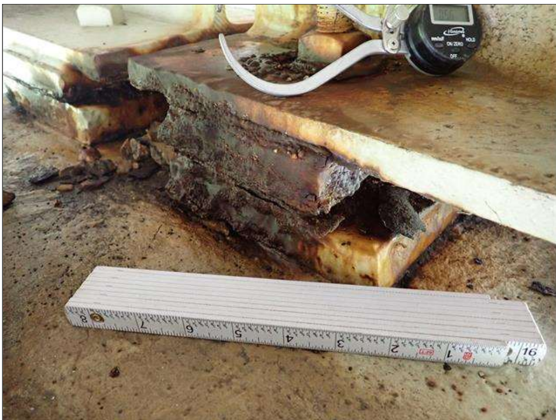
Span 2 Beam 4 - Far Bearing 4: corrosion with section loss (up to 3/16 inch deep)
