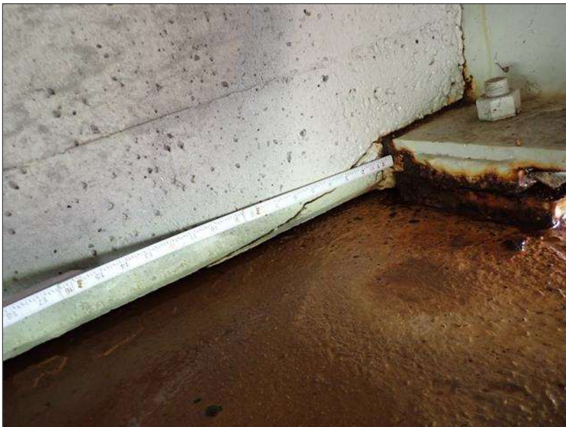
End Bent 1 Abutment: at beams 1 and 3 penetrations, diagonal cracks, up to 12 inch x 1/16 inch
