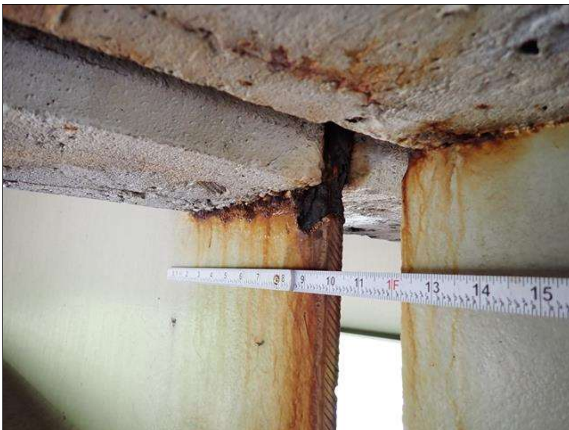
Span 3 Beam 3: at bent 2, painted over section loss/pitting: web adjacent to end diaphragm (9/16 inch average remaining x 9 inch x 1 inch)
