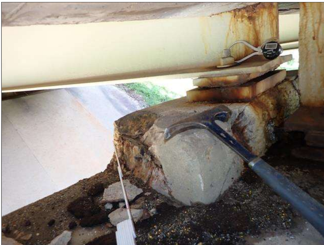
Bent 3 Cap 1: (PAR) 6 INCH X FULL WIDTH X 12 INCH X 2 INCH DEEP SPALL WITH EXPOSED REBAR WITH APPROXIMATELY 25 PERCENT LOSS, WEST FACE, IN BEAM 3 PEDESTAL.
