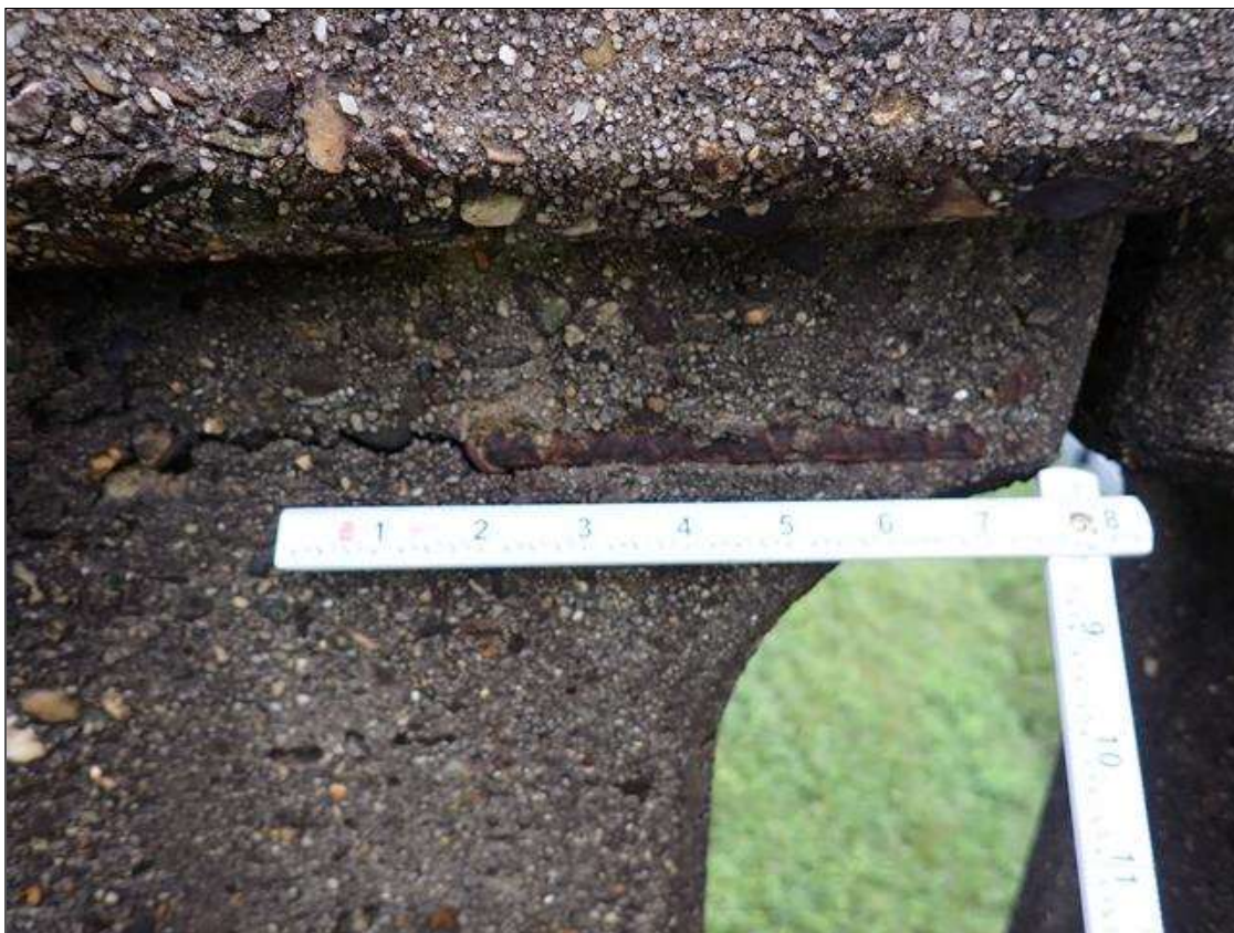
Span 1 Left Bridge Rail: UP TO 6 INCH X 3 INCH X 1/4 INCH DEEP SPALL WITH EXPOSED REBAR AT RANDOM THROUGHOUT
