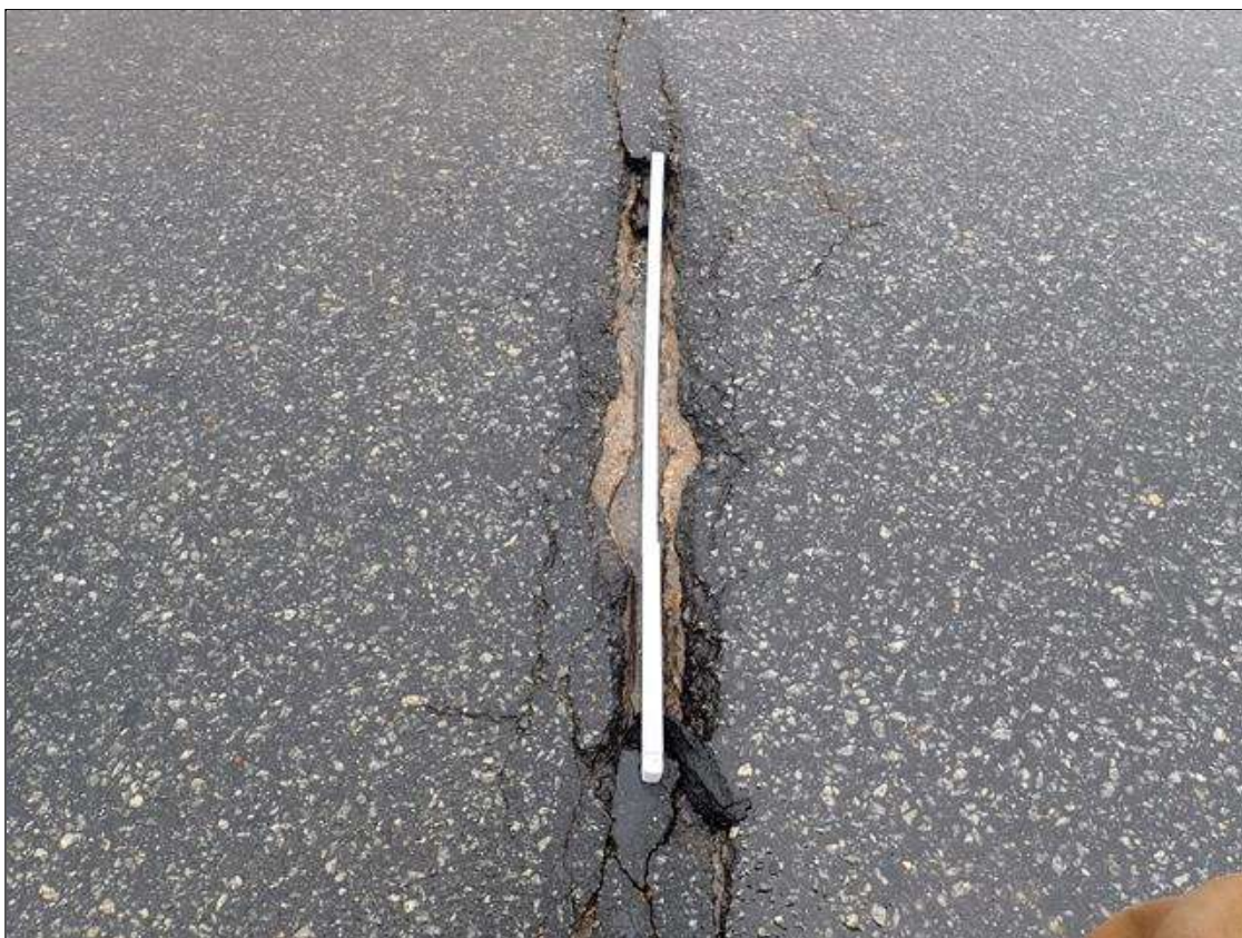
Span 2 Wearing Surface: (PAR) over bent 1, broken asphalt (full roadway width x 8 inch) with potholes (up to 32 inch x 5 inch x full depth)
