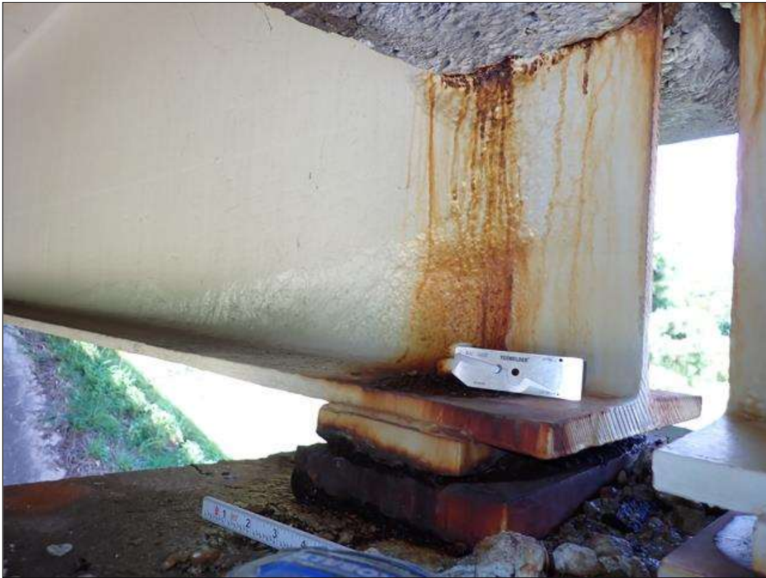
Span 4 Beam 5: at bent 3, painted over pitting: bottom flange (up to 1/8 inch deep x 3 foot); web (up to 1/8 inch deep x 5 foot x 15 inch)
