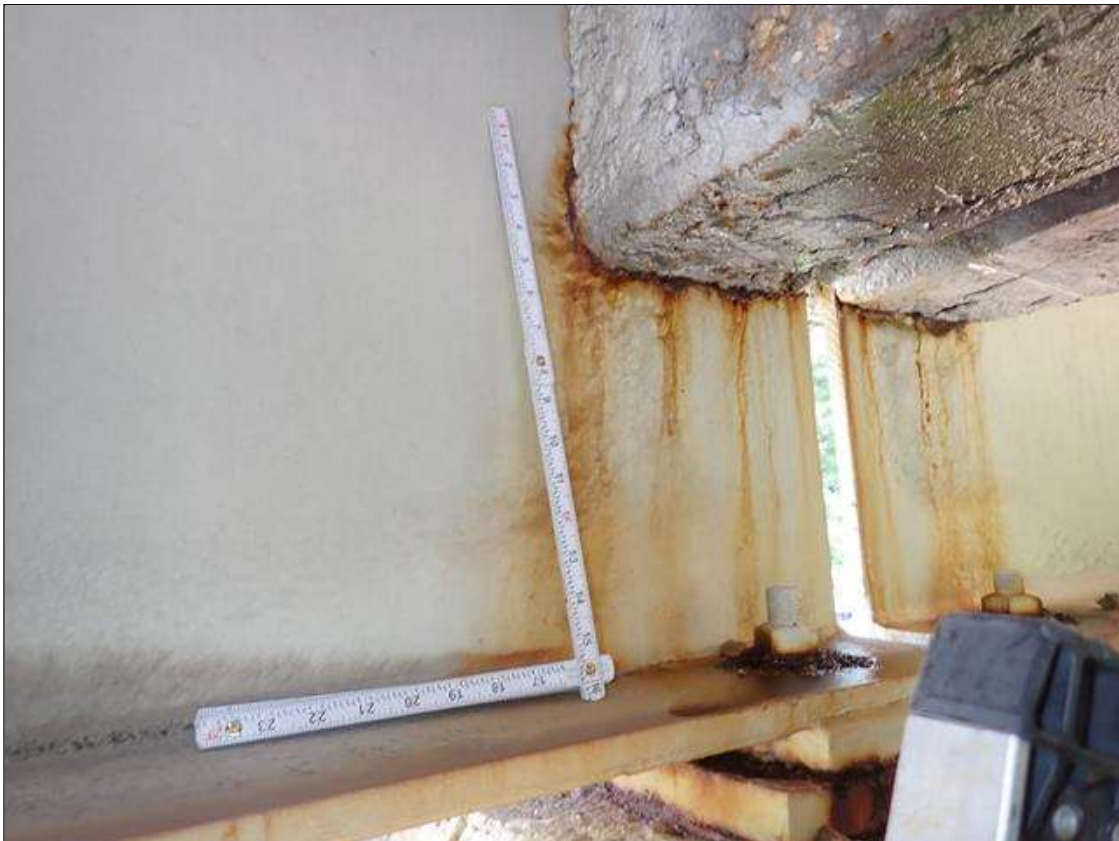
Span 3 Beam 1: at bent 3, painted over section loss/pitting: bottom flange (0.67 inch average remaining x 3 inch); web adjacent to end diaphragm, painted over pitting (up to 1/8 inch deep x 14 inch x 12 inch)
