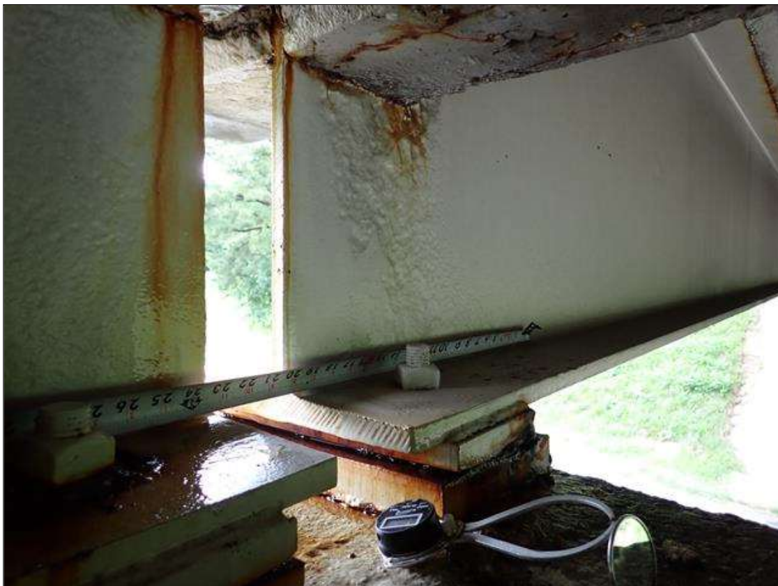
Span 3 Beam 1: at bent 2, painted over section loss/pitting: web adjacent to end diaphragm (1/2 inch average remaining x 16 inch x 13 inch); bottom flange, pitting (up to 1/16 inch deep x 16 inch) with corrosion reactivating
