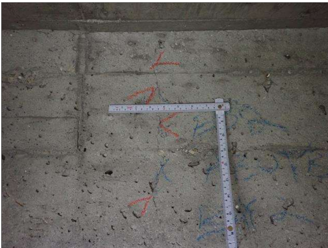
End Bent 2 Abutment: END BENT 2 ABUTMENT THROUGHOUT ALL BAYS, VERTICAL CRACKS, UP TO 2 FOOT X 1/64 INCH
